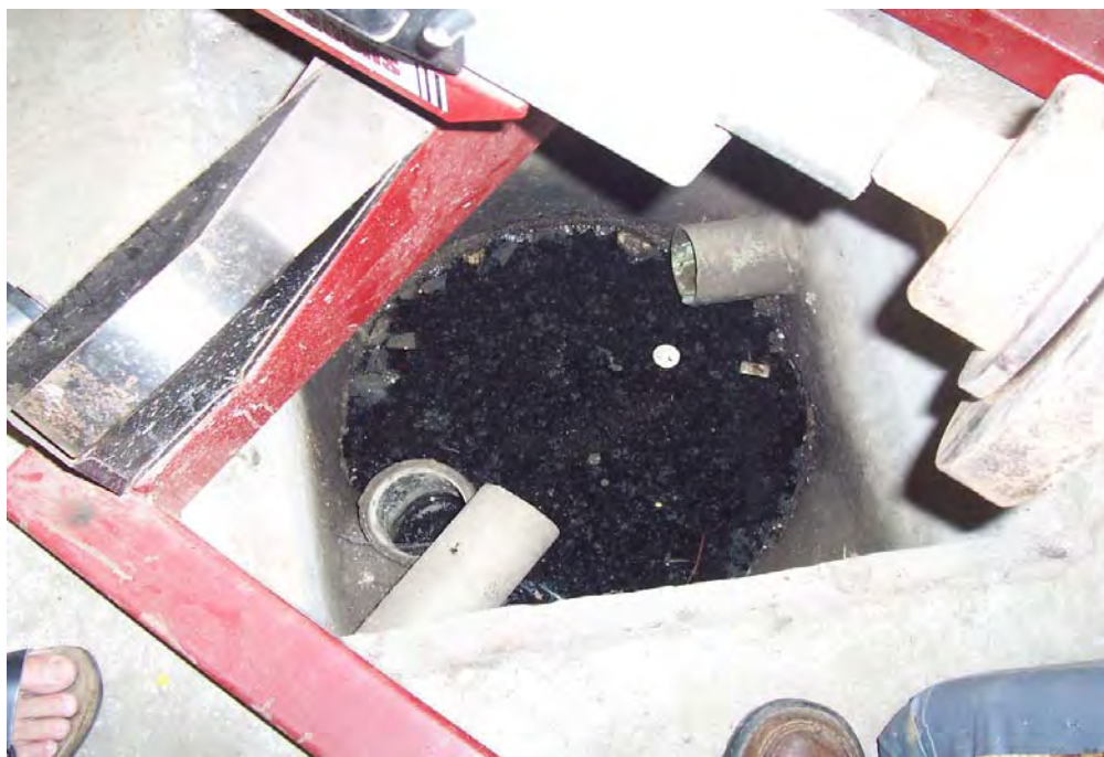
Photograph 11: Collector pit in the maintenance garage. There was no indication of oil or odours in the pit.
