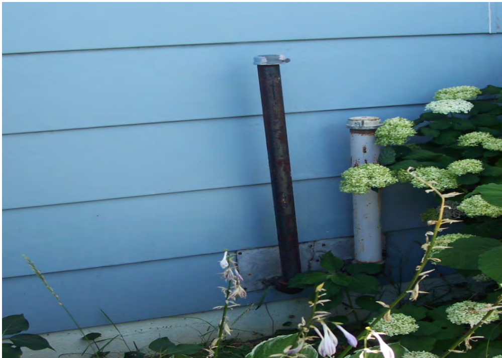
Photograph 3: Fill and vent pipe for the basement heating oil tank.
