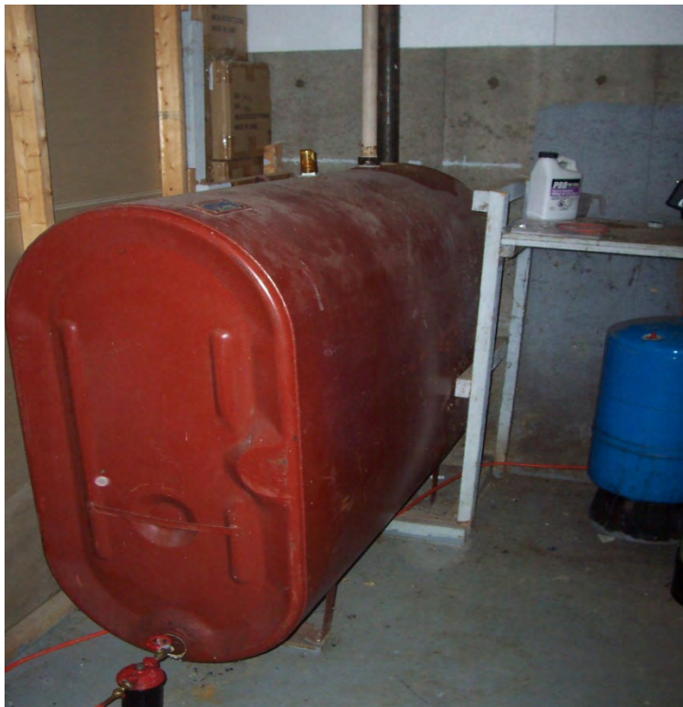
Photograph 2: Oil tank in the basement. No leakage or spills observed under the tank.
