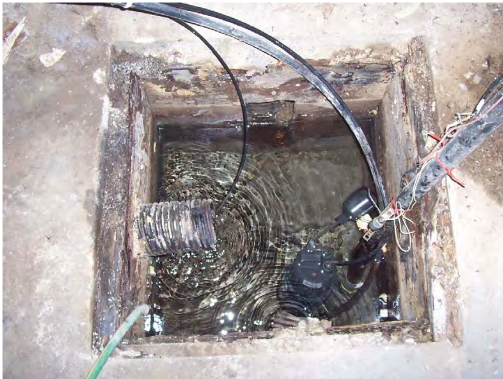
Photograph 4: Sump pit in the basement. No hydrocarbon issues with the water observed in the pit.
