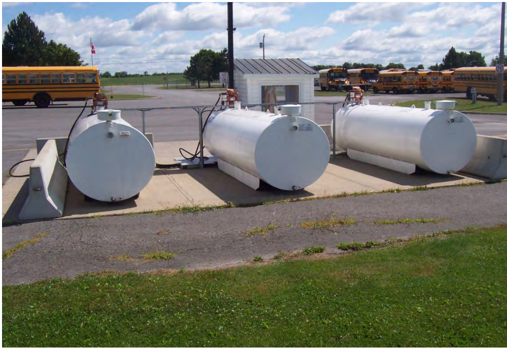
Photograph 3: Three ASTs located in the fuelling area.
