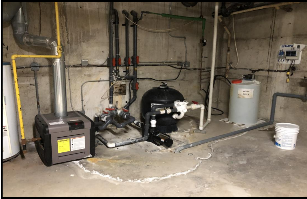
Photograph 5: View of a natural gas-fired burner, used for heating the interior swimming pool, located in the basement of the recreational amenity building.
