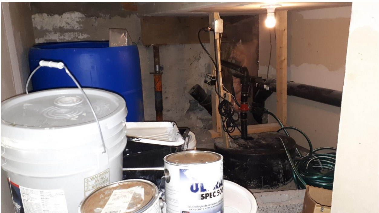
Photograph 6: View of sump pit crawlspace in the basement of the office building at 979 Wellington Street West.
