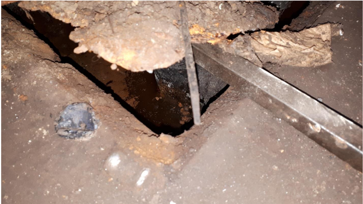
Photograph 5: View of the oil-water separator pit in the northeast corner of the service garage building.
