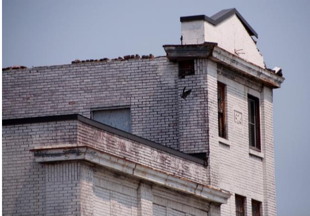
Figure 33: The gabled brick and metal parapets will be re-instated to their original form and design. The height of the parapet can be determined from period photos. The original colour of the brick is evident in areas where the paint has worn off.
