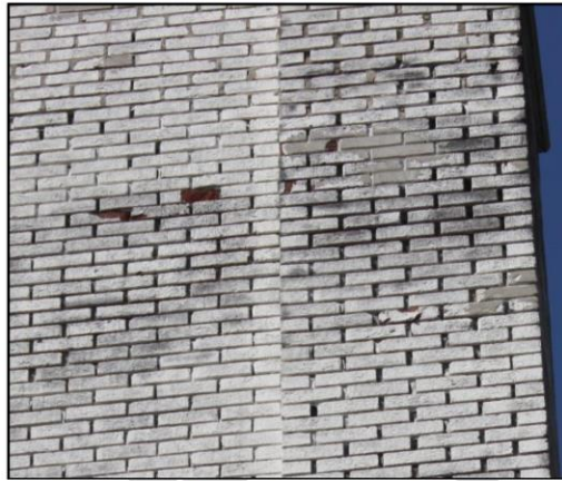
Photo 5: Typical localized area of eroded joints and face spalled bricks [JCAL 2018].
