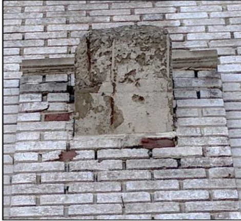
Photo 4: Typical corbel on the west elevation. Concrete and bricks are deteriorating [JCAL 2018].
