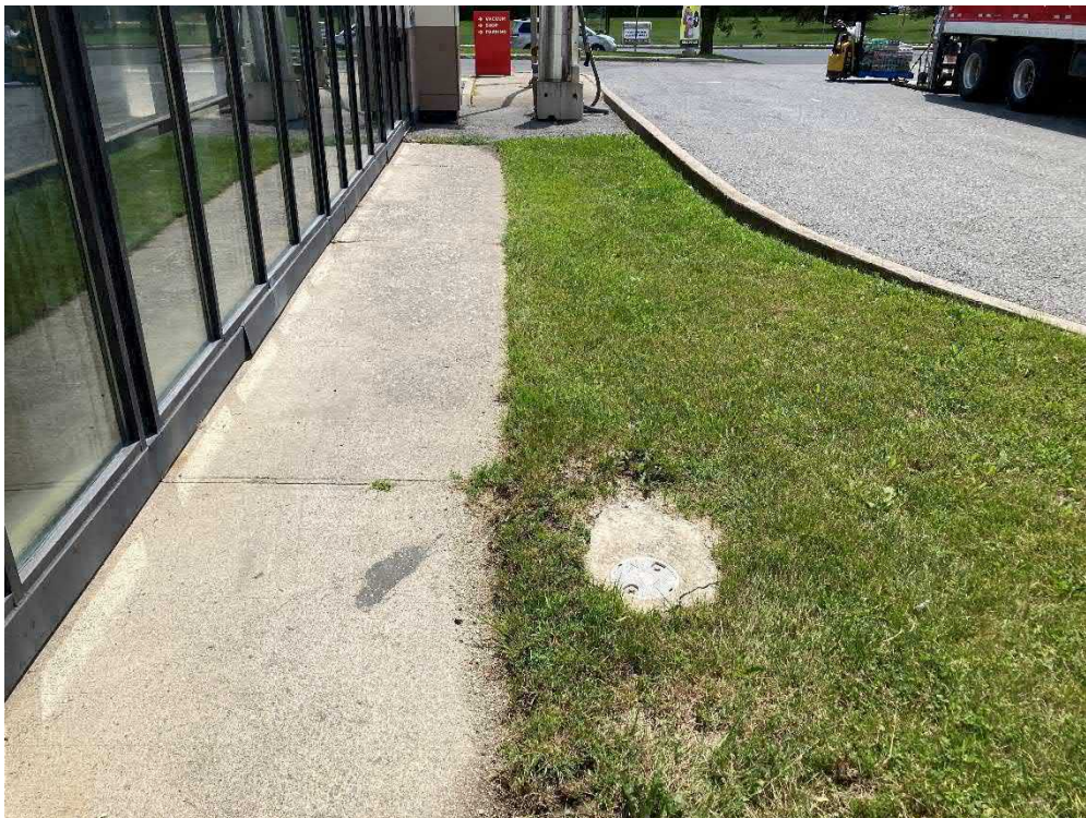
Photo 10: View of a monitoring well installed in a landscaped area west of the car wash
