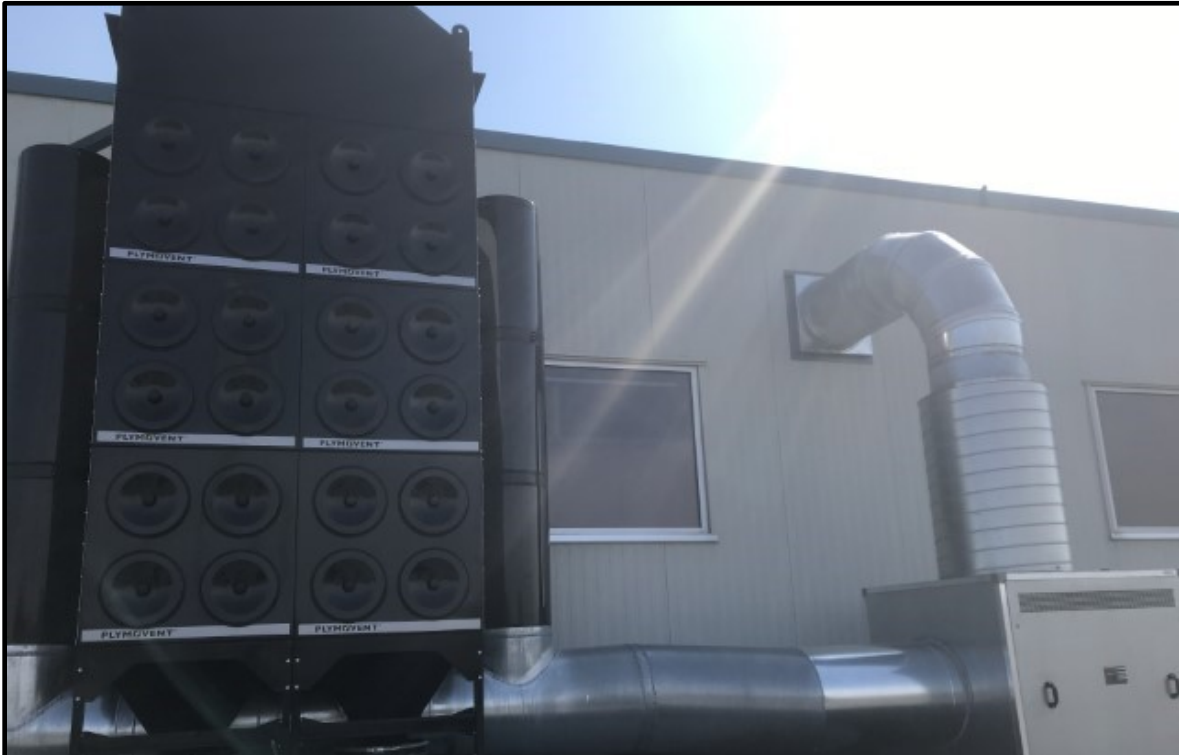
Photo 19: Central extraction fan with two drums for the collection of welding dust.
