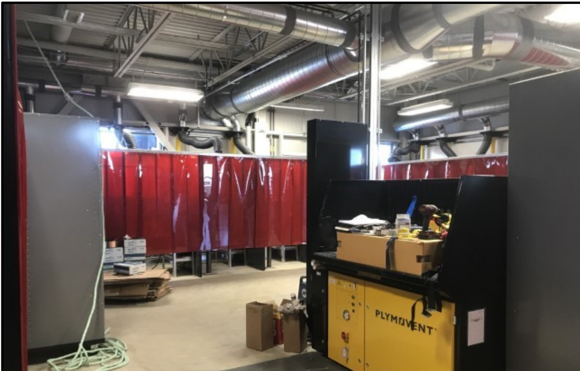
Photo 16: Welding training area with central extraction fan unit.
