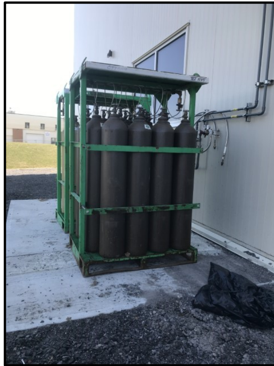
Photo 29: Photo of compressed argon cylinders secured vertically in two storage cabinets on a concrete pad, to the north of the Site building.
