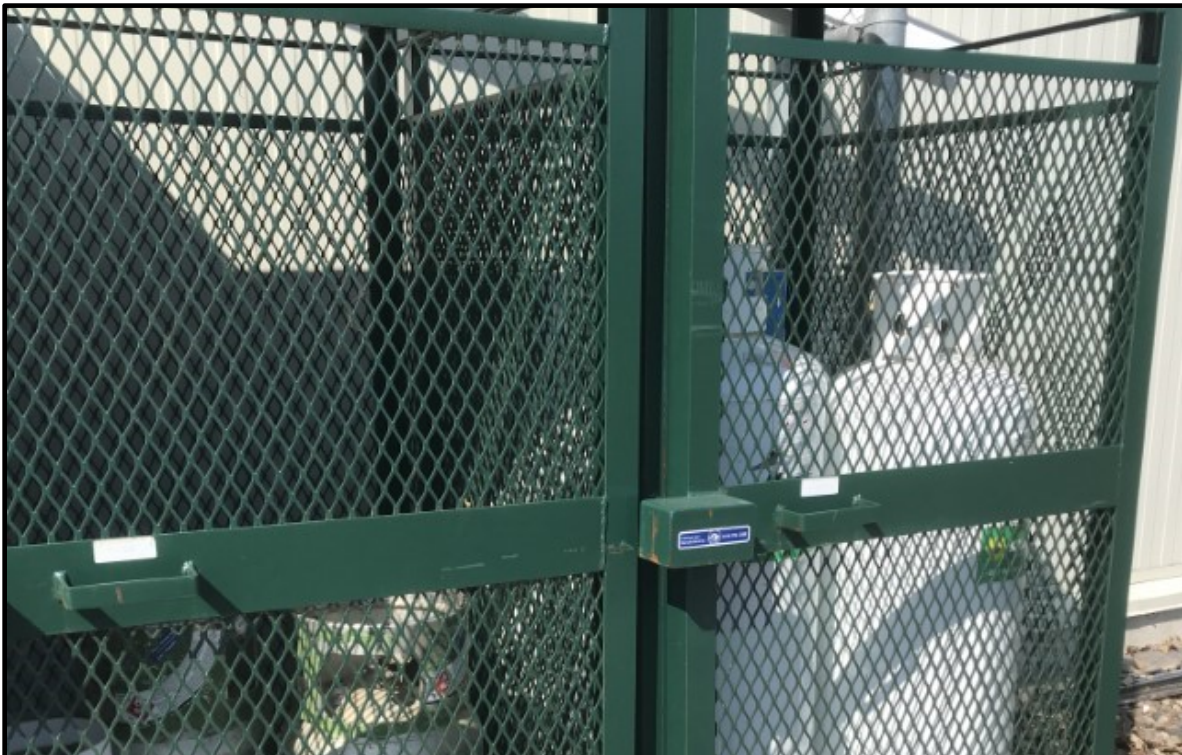
Photo 28: Photo of propane cylinders secured vertically in a storage cabinet to the east of the Site building.
