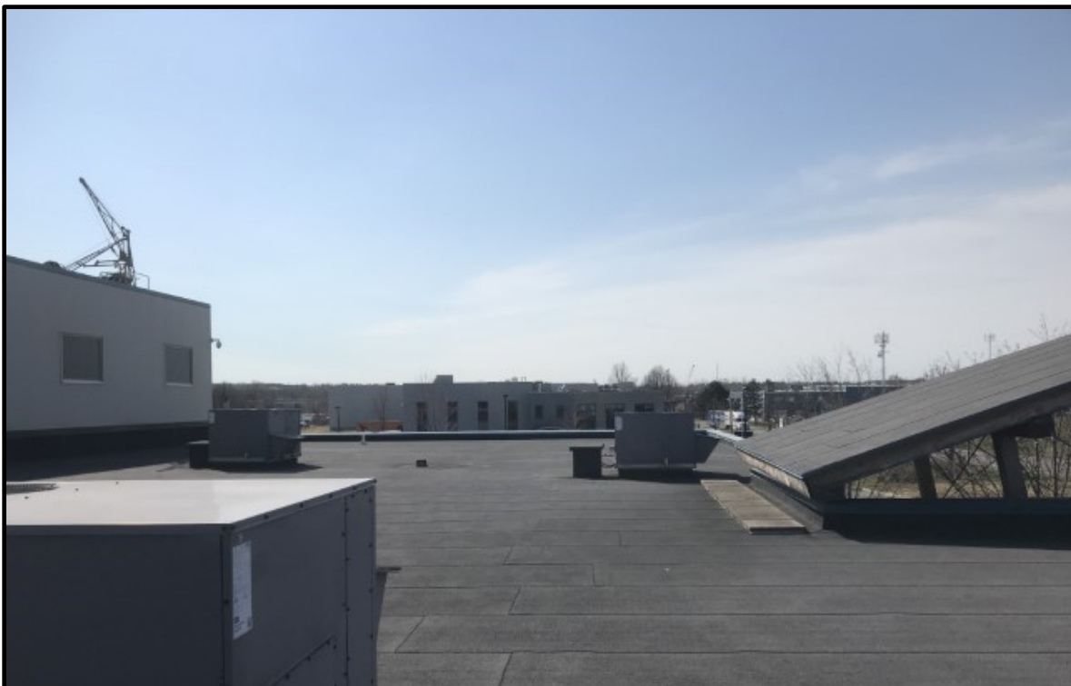
Photo 20: Rooftop view of four air handling units.
