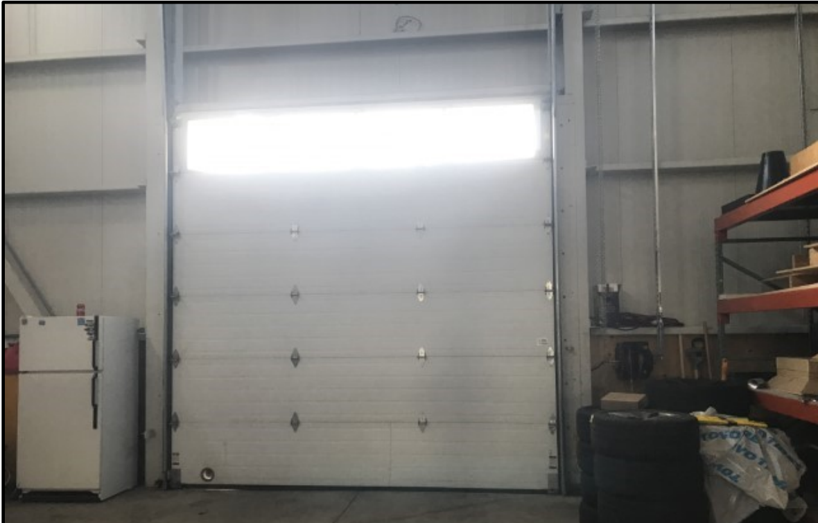
Photo 13: Electric garage door in training centre.
