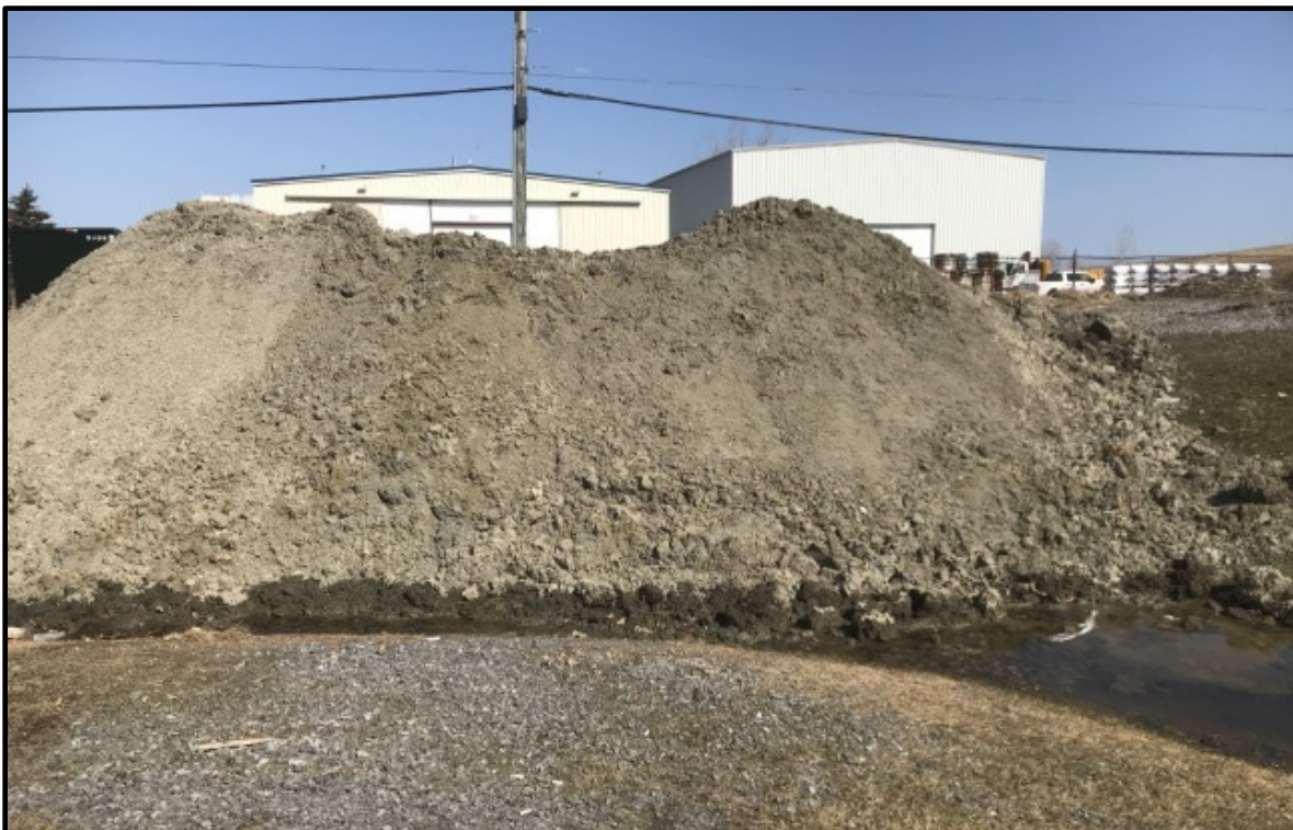
Photo 22: Photo of silty clay native material, originating from the property directly to the north of the Site, excavated during the installation of the onsite transformer.
