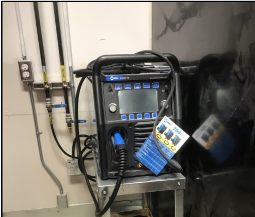
Photo 17: Individual workspace for welding training with argon piping.
