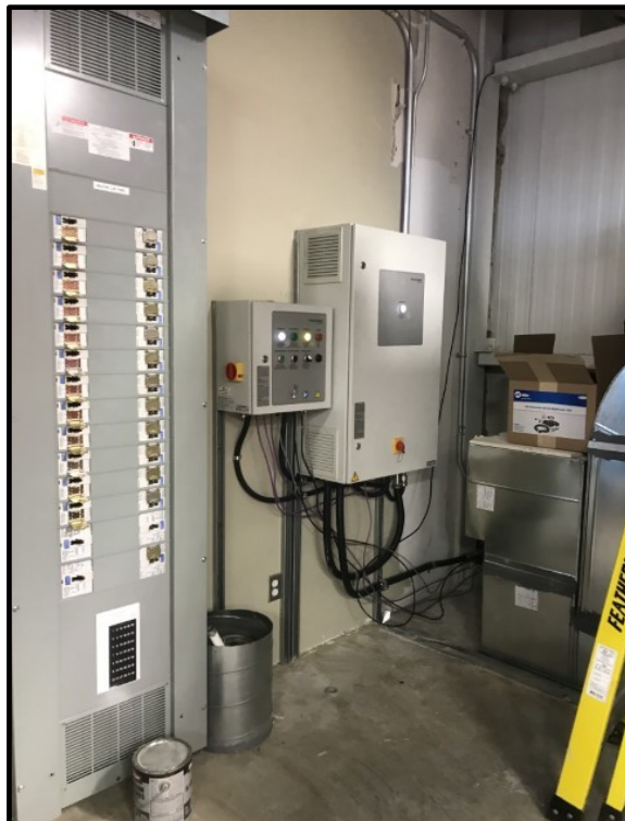
Photo 18: Electrical unit in welding training area.
