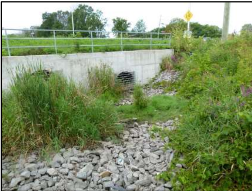
Photograph 15: Stormwater pipes outletting to the southern stormwater swale (Tributary #4) (facing west towards March Road). Note the lack of surface water (August 14 th , 2017).
