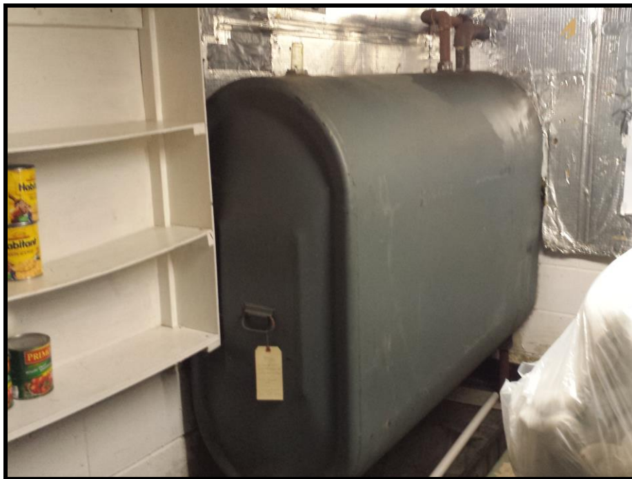
Photograph 6: View of an oil tank, located in the basement of the occupied residence situated on 4055 Russell Road (addressed 3995 Russell Road).
