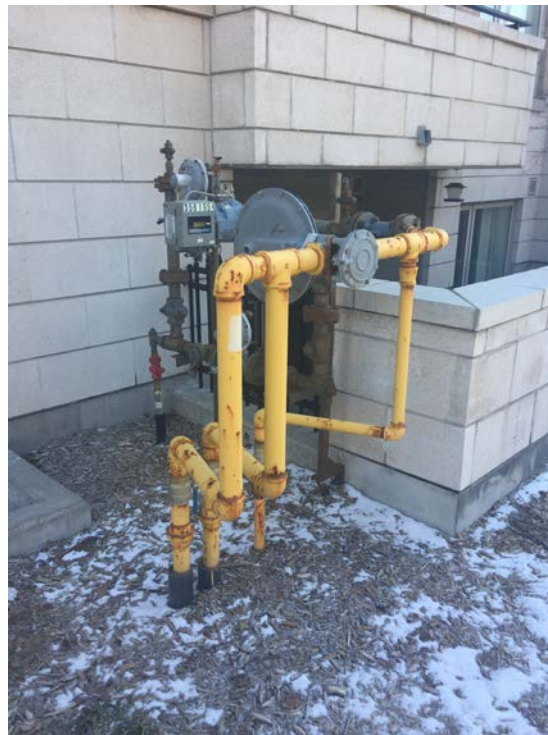
View of natural gas meters for residential building located immediately west of 32 Florence Street
