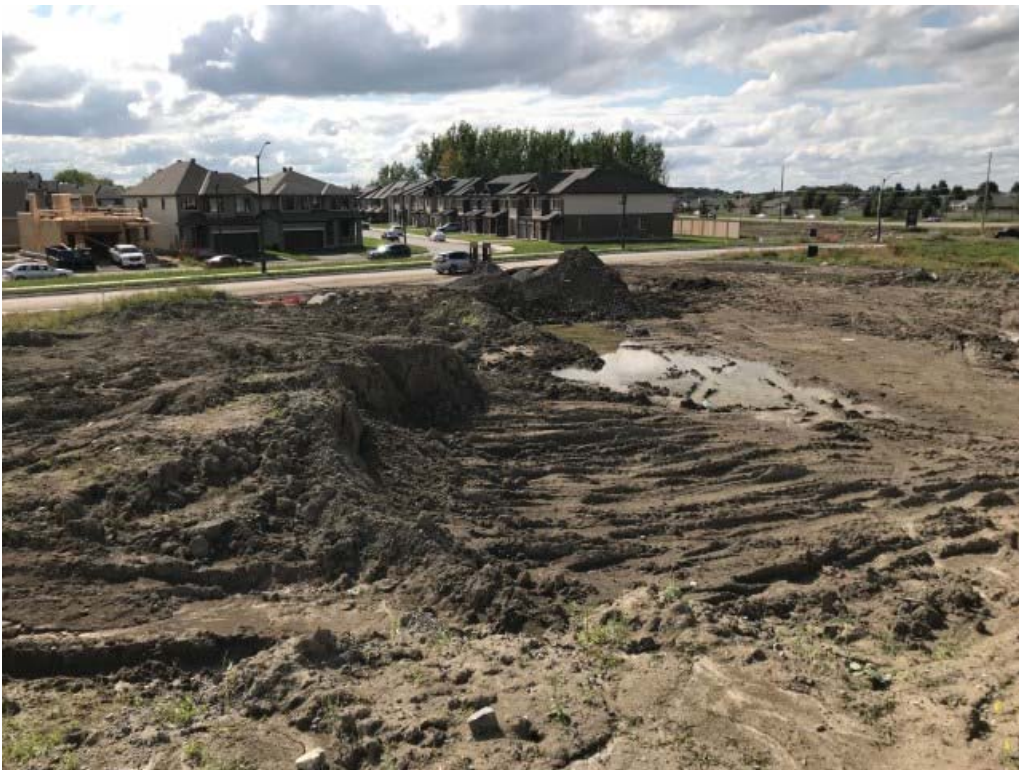
Photo 4: View of disturbed soil on Site, facing west.
