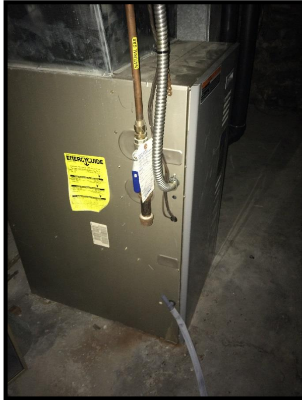
Photograph 5: View of the natural gas forced air furnace.
