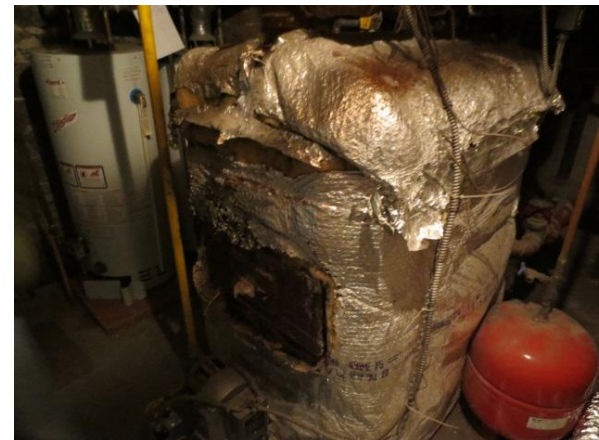
4. View of the natural gas fired boiler located in the basement of building on the Phase One Property.
