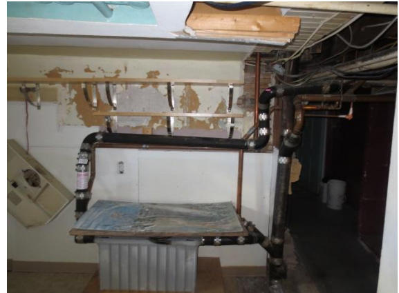
8. View of the basement of the building on the Phase One Property.
