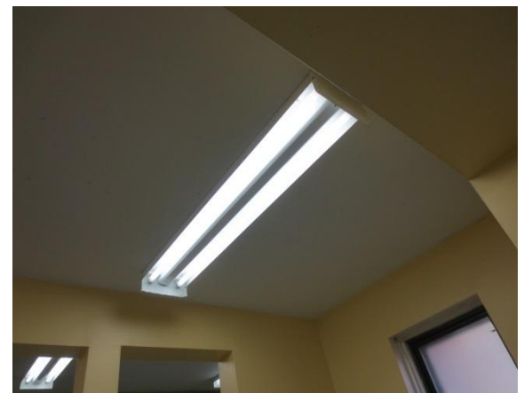
6. View of fluorescent lights observed in the building on the Phase One Property.
