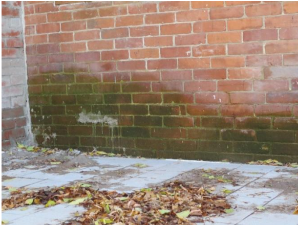
9. View of water staining observed on the exterior of the building on the Phase One Property.
