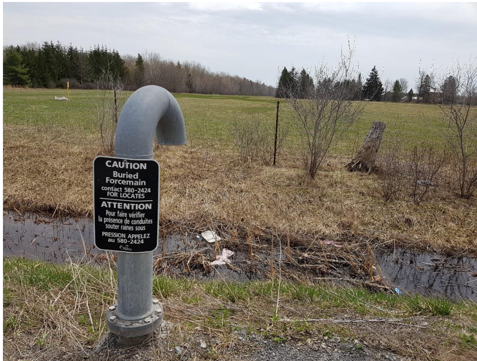
Photo 3: Buried Force-main adjacent to Franktown Road
