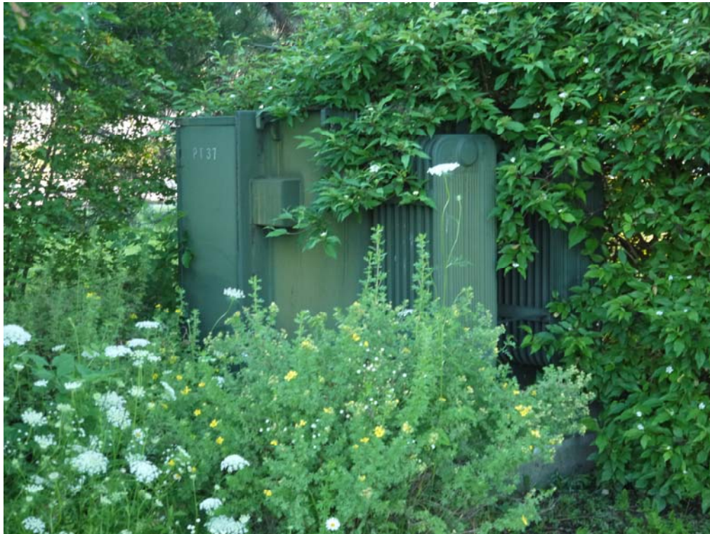
Transformer adjacent to northeast corner of site (located at 2355 St Laurent Boulevard) with possible PCB containing equipment.
