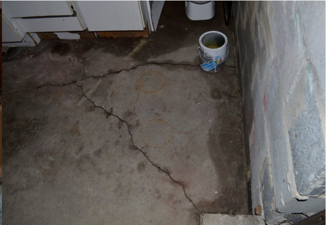
Typical cracked basement slab and water infiltration.
