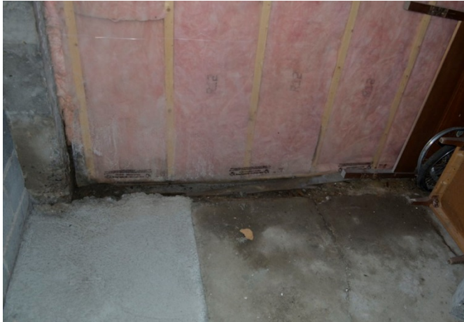
Evidence of repairs and water infiltration at cracked basement slab. Note new slab infill on the left side.
