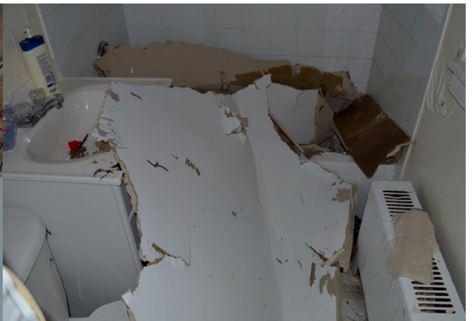
Collapsed drywall ceiling due to water infiltration.
