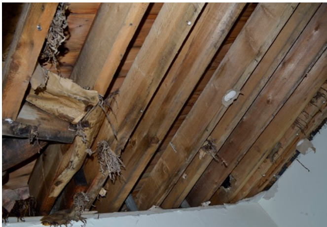
Exposed floor joists at collapsed drywall ceiling due to water infiltration.
