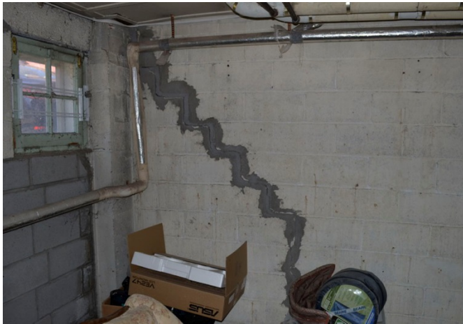
Evidence of repairs at extensive cracking in basement foundation wall.
