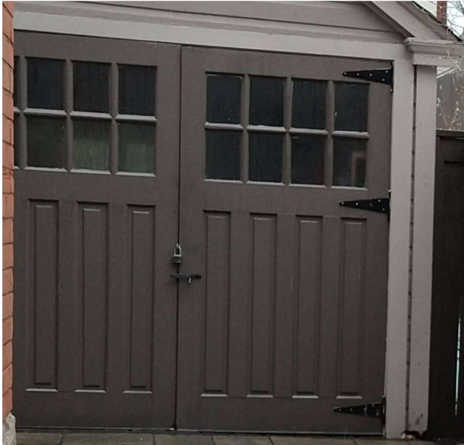
Fig. 21. Garage doors were replaced by then owner in the 1990's as original doors were finished. Doors swing sideways and cannot be opened during the winter months due to frost heave of the driveway in front of the garage. Doors were cut 2 inches last year to attempt to correct issue, but another 2 inches would need to be cut from the bottom so that they could swing open properly.
