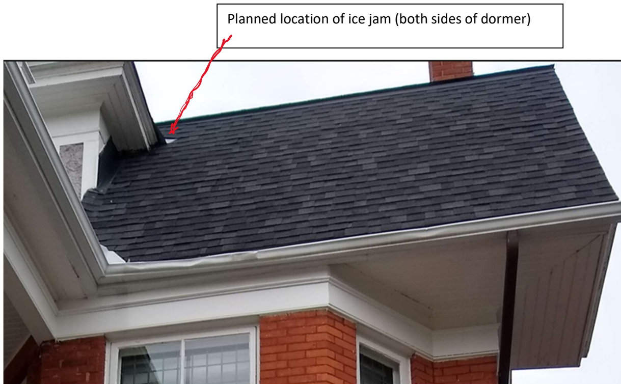
Fig. 16: Eavestroughs damaged from ice sliding down from above
