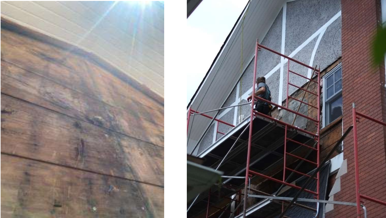
Fig. 6 and Fig. 7: Exposed boards after stucco panels were removed
