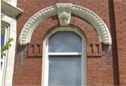
Figure 12: Moisture staining below window lintels
