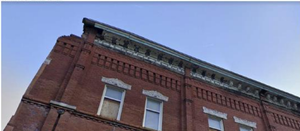
Figure 19: Missing cornice brackets, and general deteriorated condition on the north façade.
