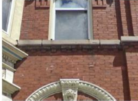
Figure 13: Open skyward facing joints on the stone stringcourse with stained and eroded brick dentils below.
