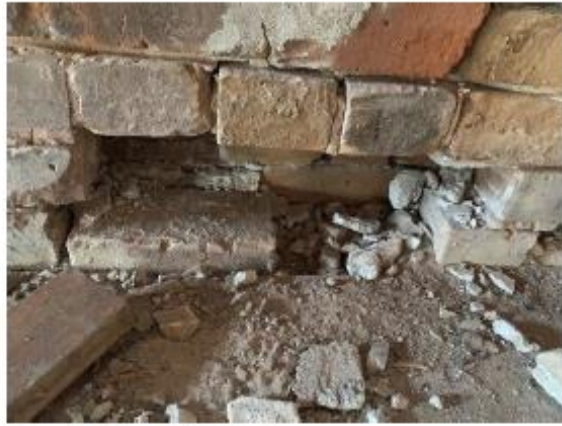
Figure 40: Debonded brick wythes.
