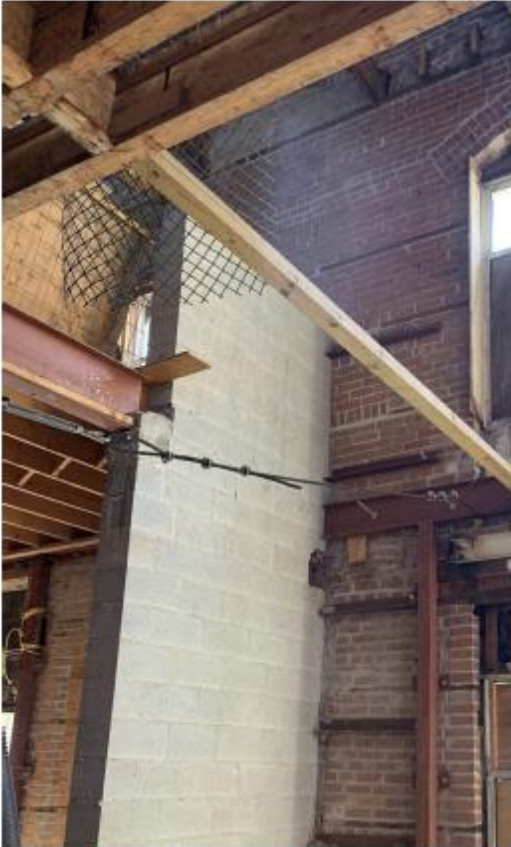
Figure 47: Second floor steel beam is supported at the edge of the wall.
