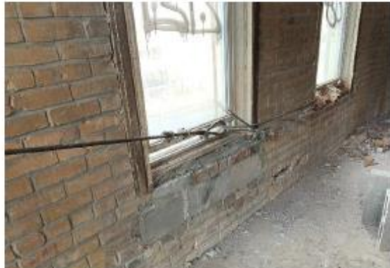
Figure 42: Steel cable between brick pier and window.
