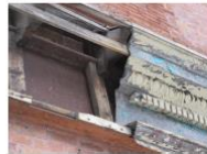
Low Level Cornice to be Replaced
