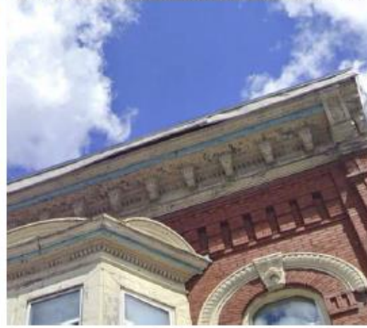
Figure 18: Separated fascia, deteriorated cornice and frieze.
