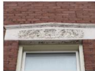
Precast Stone Window Headers to be Restored
