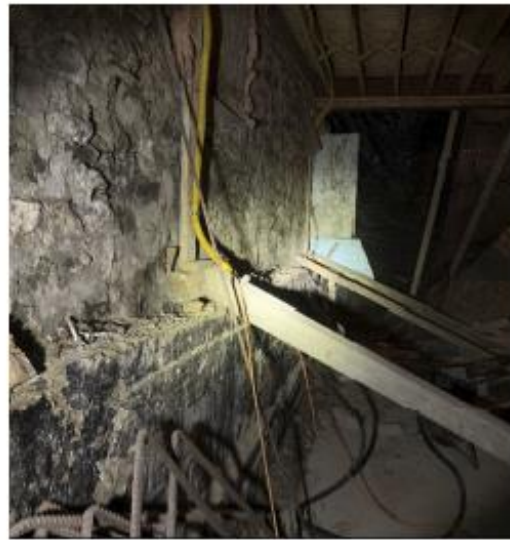
Figure 50: Cracks in the concrete foundation wall.
