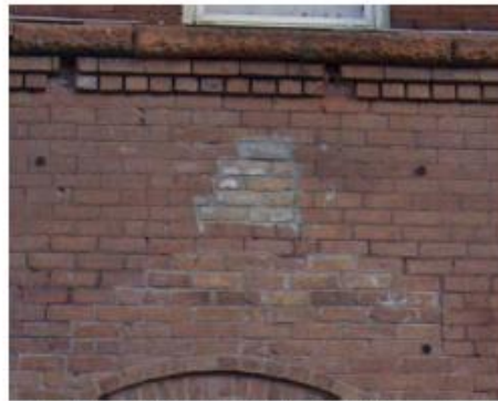
Figure 7: Incompatible previous repair above north façade door and deteriorated brick corbelling above.
