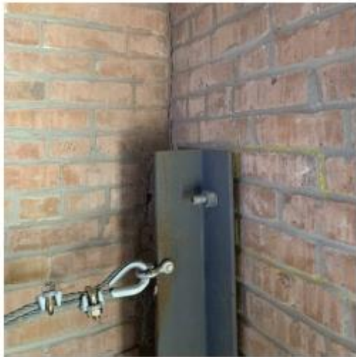
Figure 43: Vertical structural crack at the southwest corner.
