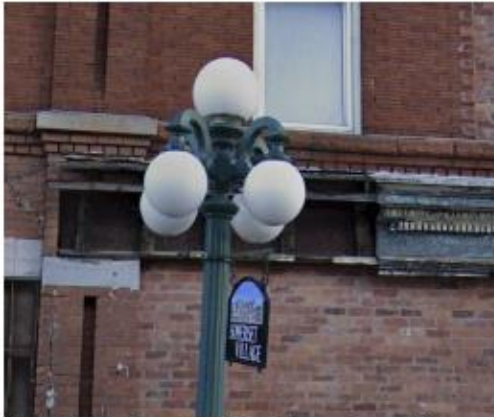
Figure 15: Missing section of first floor cornice and frieze.
