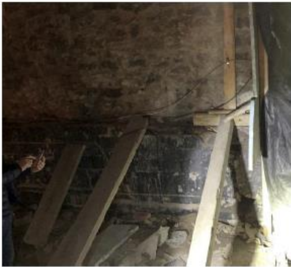
Figure 49: Deteriorated condition of the north foundation wall.
