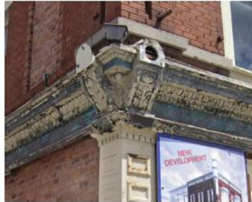
Figure 16: General deteriorated condition of first floor cornice.
