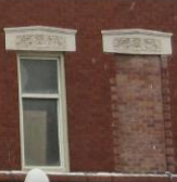
Existing windows and terracotta lintels at 2nd level. Existing window masonry brick infill to be removed and replace with new window.
