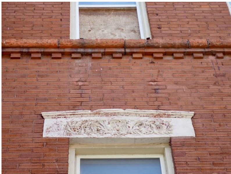
Figure 10: Detail view of the second-floor sill course on the Somerset Street elevation. Note the rusticated terracotta sill (belt) course above the brick dentil band and the painted terracotta window lintels. Source: Heritage Ottawa / Archives Ottawa.
