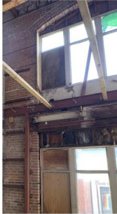
Figure 48: Gaps around the window.
