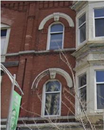
Figure 20: Missing arched metal lintel on west façade.
