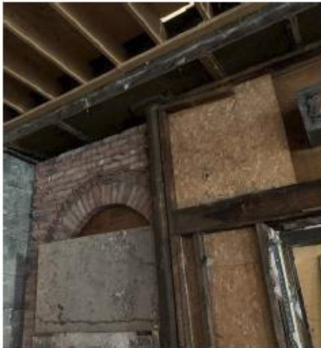
Figure 29: west façade window blocked with fiberboard.
