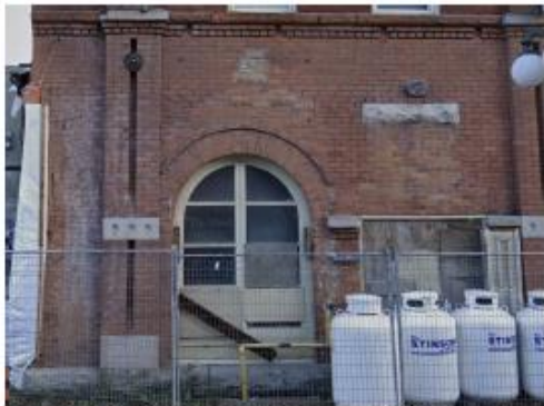
Figure 6: Brick efflorescence and debonded joints above the window on the north façade.
