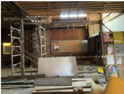
Figure 37: Deteriorated brick pier.
