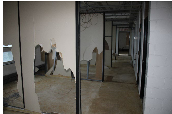
Photo 54: Representative sixth storey hallway with damaged partitions
