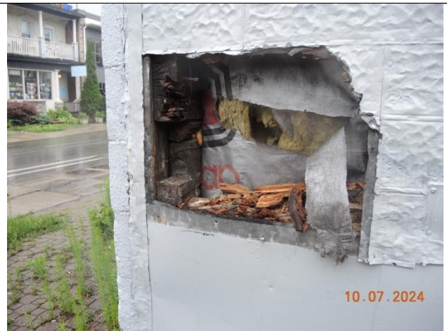
Photo 10: Advanced decay in exterior walls at opening in the cladding on East wall.
