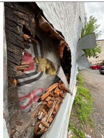
Photo 12: Remains of deteriorated wall are visible piling up at the base of opening in the East wall at the Southern edge.
