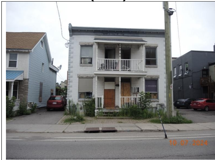
Photo 1: Front (South) façade. Two-storey deck appears to have settled.
