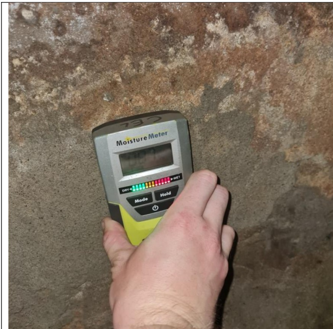
Photo 19: High moisture content near base of foundation wall (87%)
