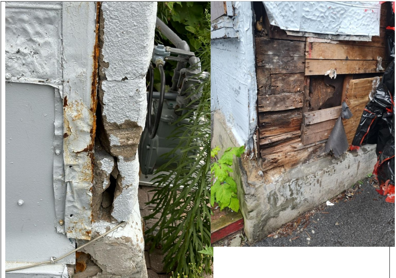
Photo 5: Cladding detaching from structure at South-West corner.
