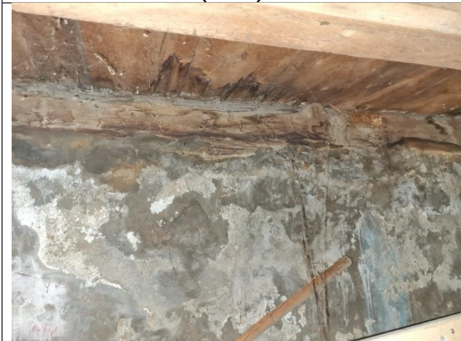
Photo 21: Decayed and stained wood structure on top of foundation wall.
