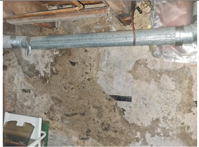
Photo 24: Severe scaling of the wall.
