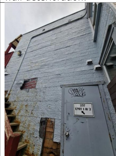
Photo 8: Bulging and peeling of existing cladding on West wall.
