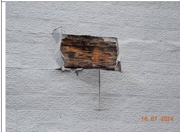
Photo 11: Advanced decay in exterior walls at opening in the cladding on East wall.
