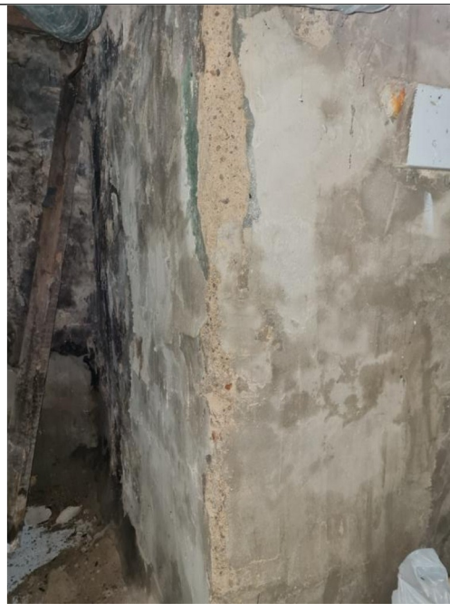
Photo 20: Deterioration of foundation wall.
