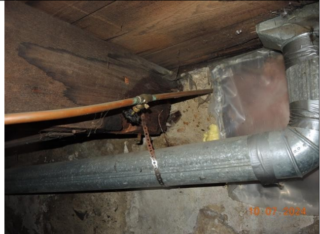
Photo 16: End of beam deteriorated due to rot. Beam has lost all connection to foundation wall.
