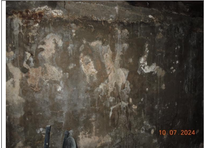
Photo 23: Crack and discolouration in foundation wall.
