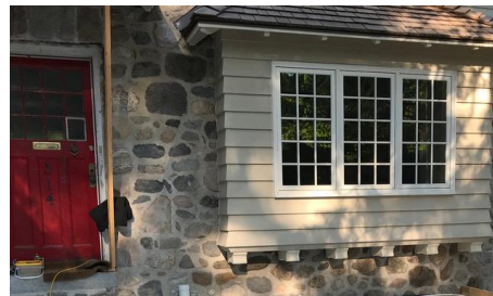
Figure 2-A: Before and After Details of the deterioration of the siding and trim around windows Source: G. Statler
