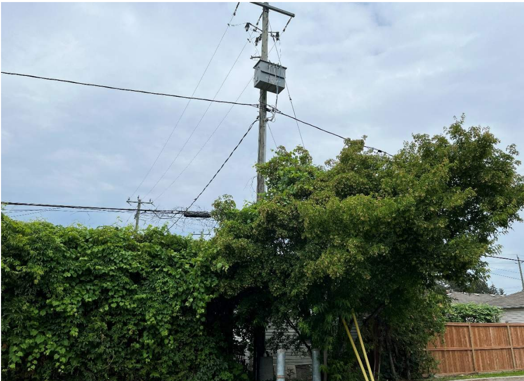
Photograph 4: Pole-mounted transformer along western property limits.
