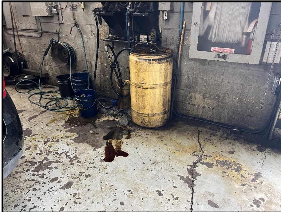
Photograph 3: View of the interior waste oil drum in the southern portion of the service bay area.
