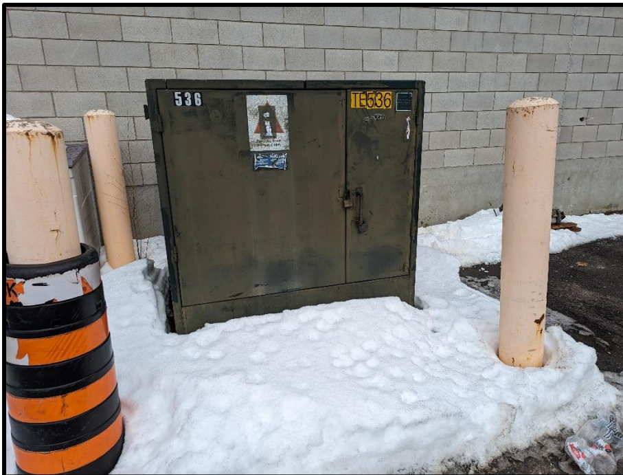
Photograph 18: View of the exterior pad mounted transformer.
