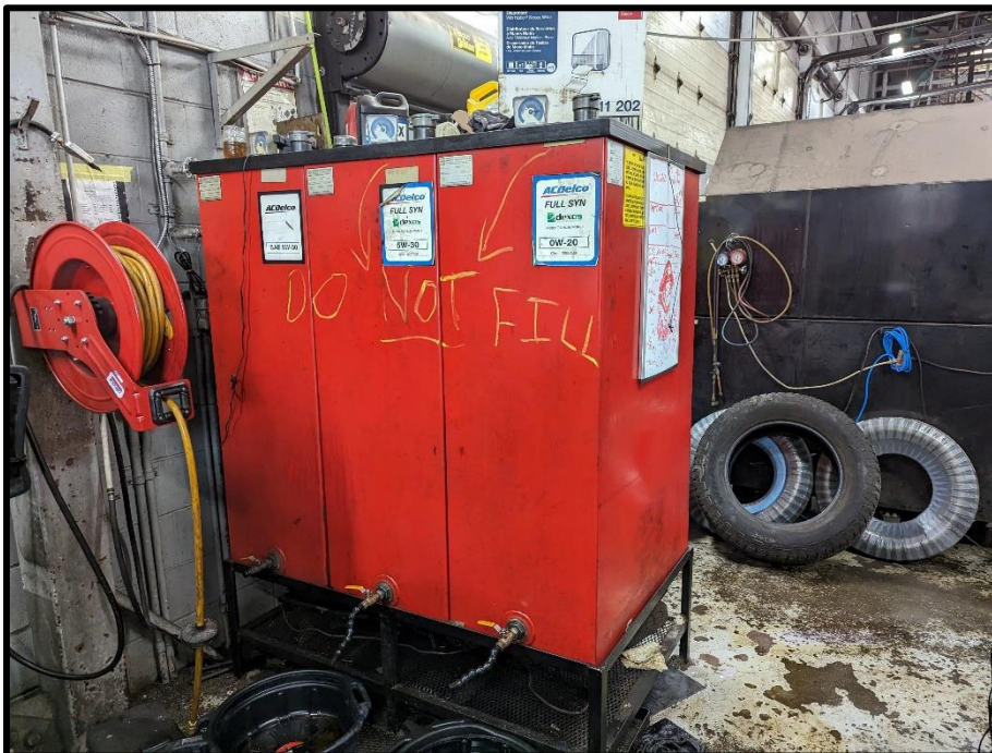
Photograph 14: View of the 3x attached motor oil ASTs along the western building face.
