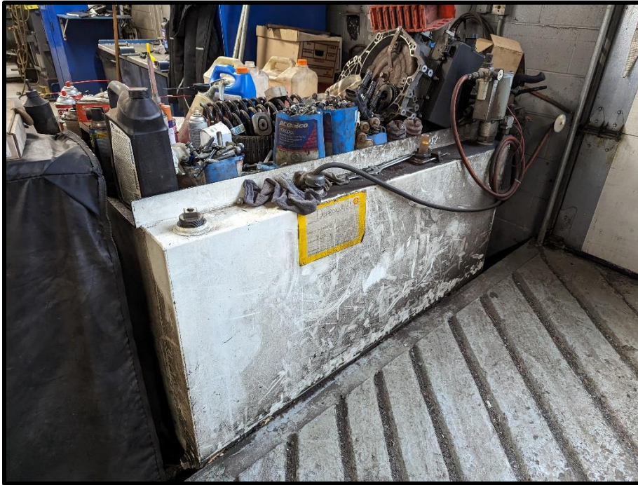
Photograph 11: View of the bench style transmission fluid AST.
