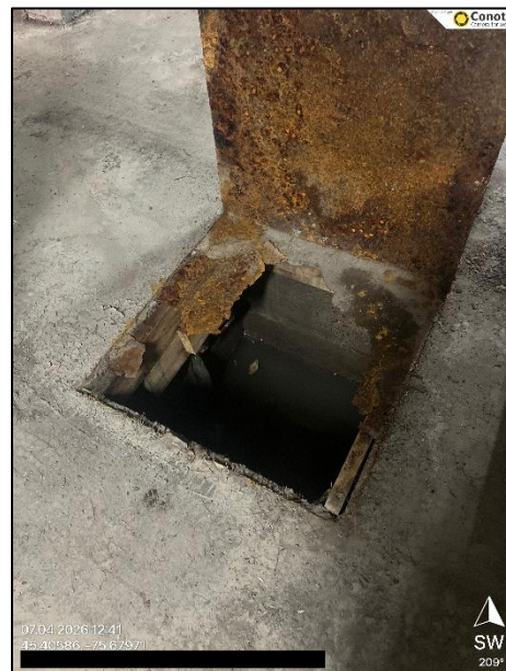
Sump observed in the mechanical room in the western portion of the on-site residential building
