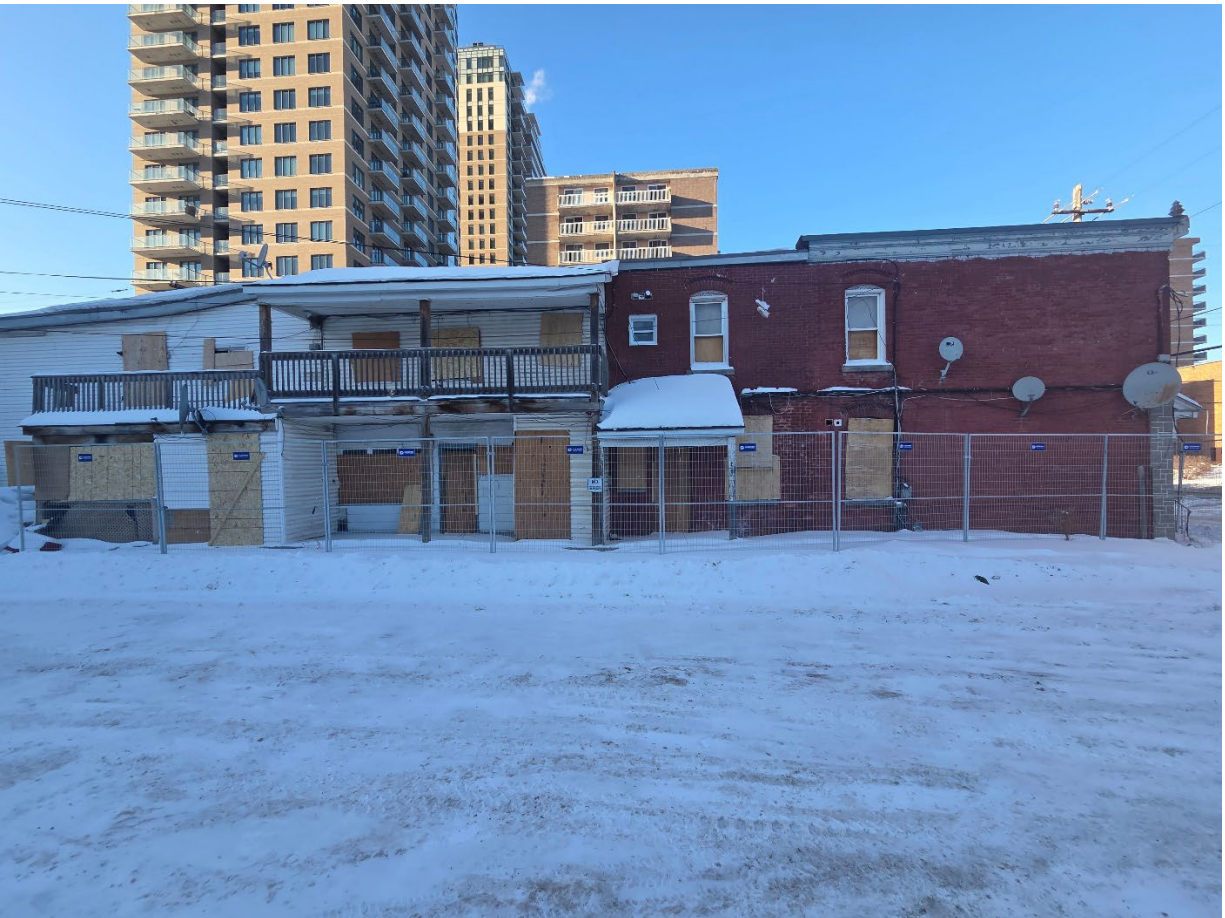
Photograph 4: View of the of the east portion of the Phase One Property looking north. View shows the vacant residential rooming house building at 122 Forward Avenue and adjacent parking area to the south.
