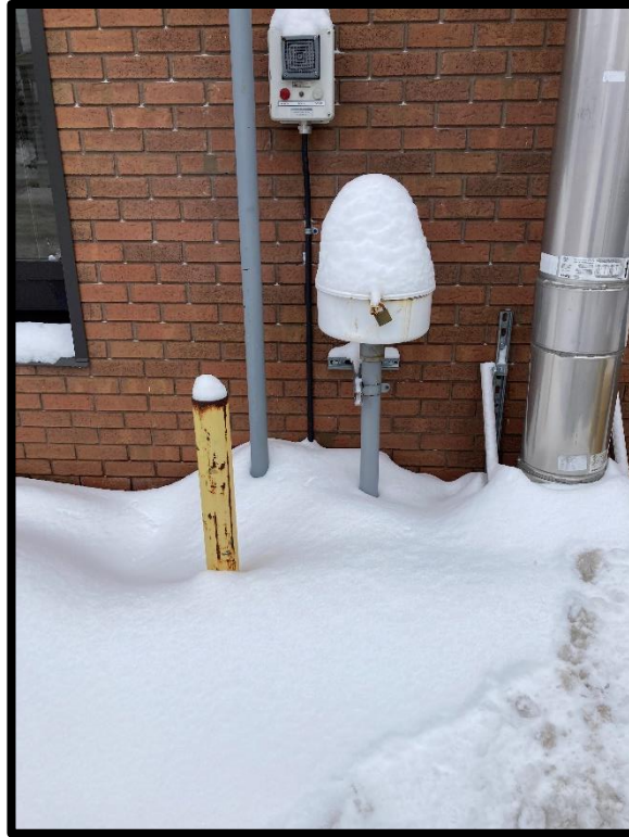
Photograph 3: View of the vent and fill pipes along the back wall of the 50 Bayswater Avenue office building, facing east.
