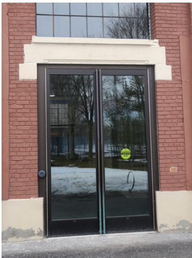
Deteriorated base on east elevation of exhibition hall (ERA 2023)
