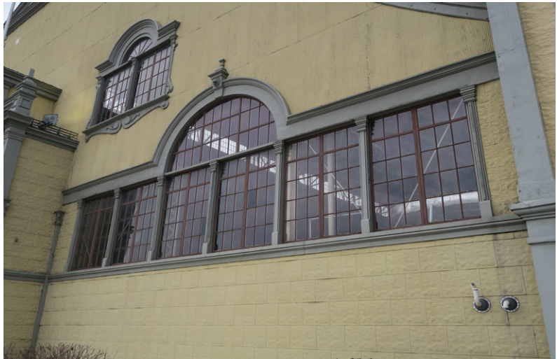
Northeast lower windows. Note dry/split wood in window frames (ERA 2023)
