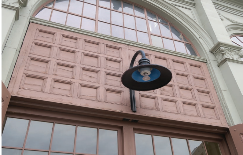
Original panelled transom over west entrance main doors. Note dry/split wood in panels (ERA 2023)
