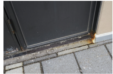
Rust damage on the bottom of the doors on the east elevation (ERA 2023)
