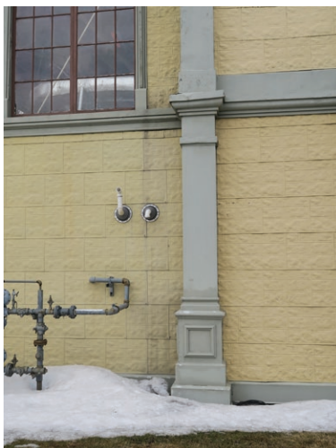
Northeast turret: damaged sheet metal capital detail and base (ERA 2023)
