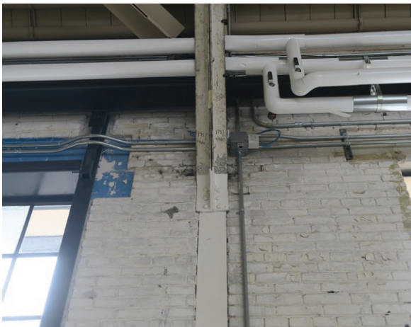
Deteriorating brick walls on the west wall of the exhibition hall at the truss (ERA 2023)
