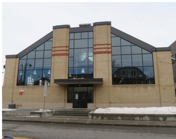
Mild efflorescence under windows of north elevation (ERA 2023)
