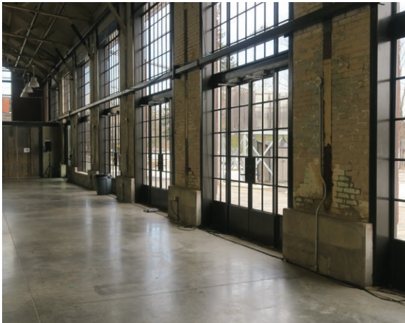
Deteriorating brick walls on the east interior elevation of the exhibition hall (ERA 2023)
