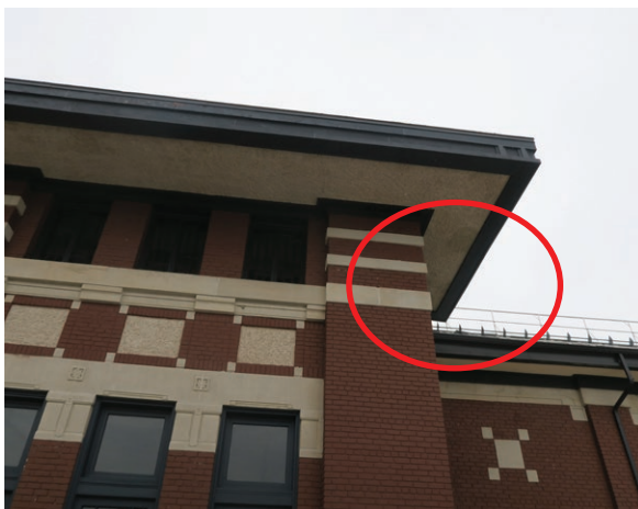
Sagging corner of the flat roof on the southeast corner of the entrance hall (ERA 2023)
