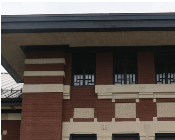
Missing stone window apron on west wing of the entrance hall (ERA 2023)
