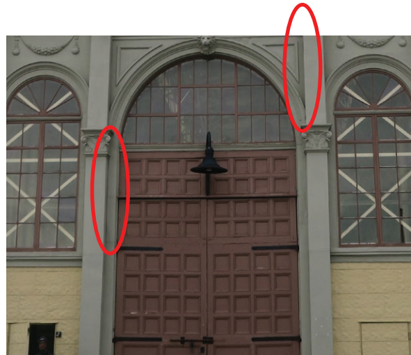
East entrance pavilion: dented metal around the doors and windows (ERA 2023)
