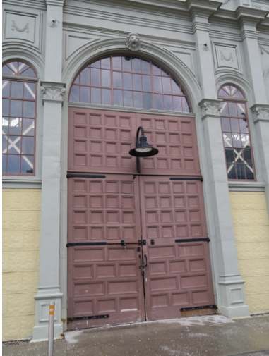
North entrance pavilion doors. Areas of dry/split wood and gaps are noted (ERA 2023)
