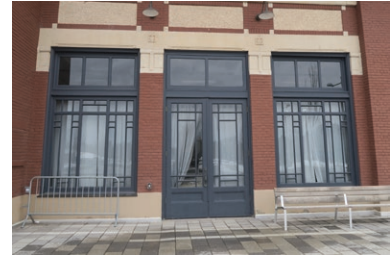
Dry and cracking wood doors on the south elevation of the entrance hall (ERA 2023)
