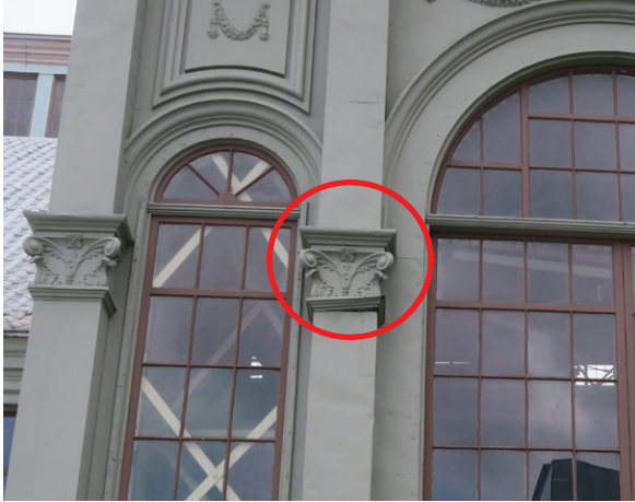
North entrance pavilion: damaged sheet metal capital details from ice and snow impacts (ERA 2023)
