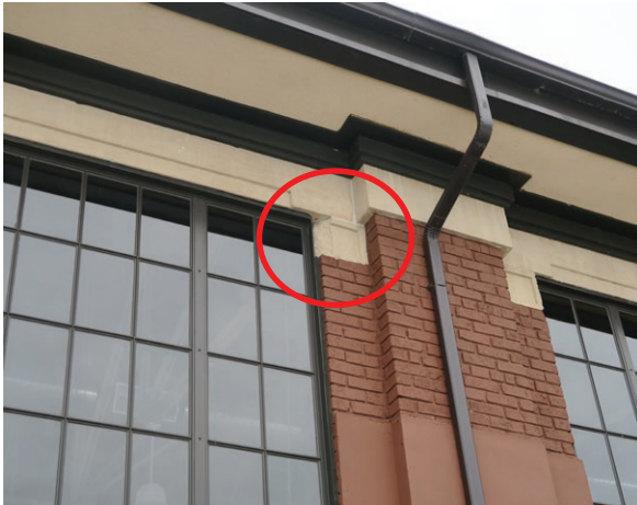
Chipped stone detail on east elevation (ERA 2023)
