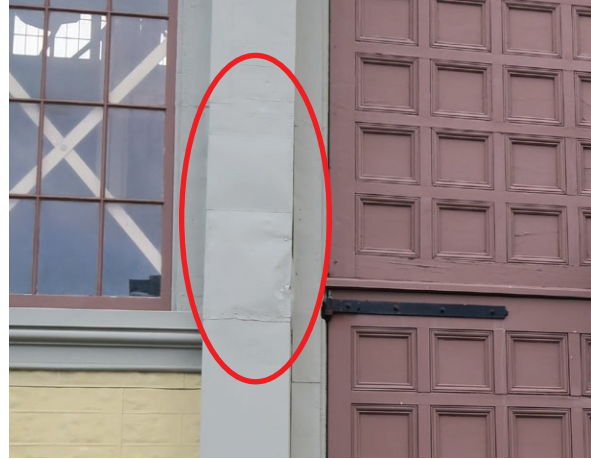
North entrance pavilion: rusted base and dented metal on pilaster adjacent to doors (ERA 2023)
