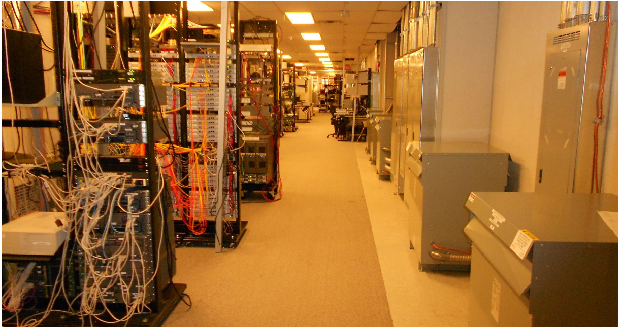
Photo 18 View of typical server lab; dry transformers observed.
