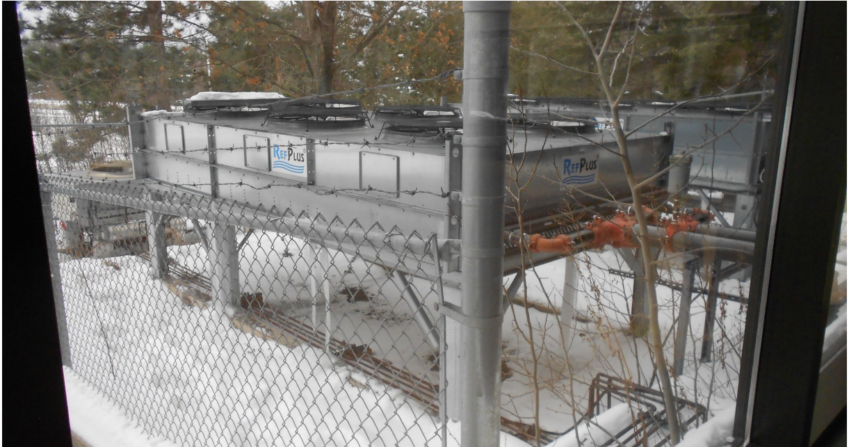
Photo 25 Typical exterior heat exchanger system (glycol or refrigerant).
