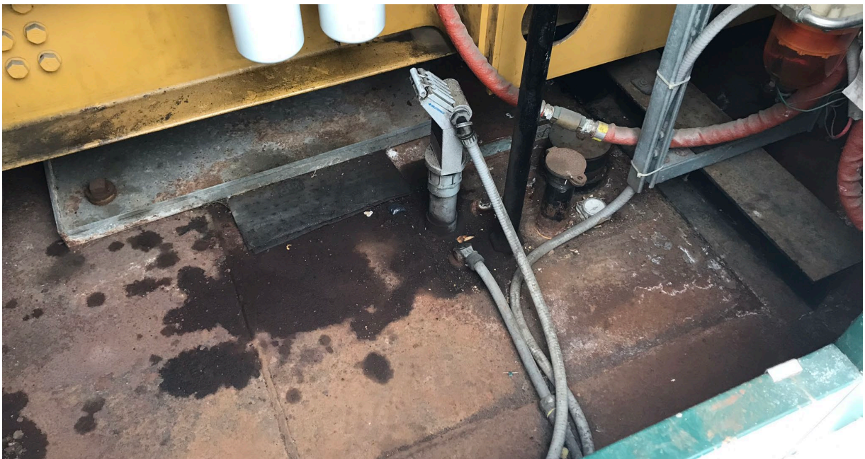
Photo 26 Evidence of drips/staining below generator (on top of decommissioned flat tank) in outbuilding located in the northeast portion of the Site.
