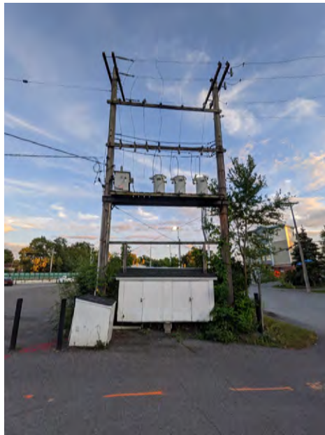
Photo 10 – Suspended transformers, westside parking lot entrance, adjacent to New Orchard Ave, facing south
