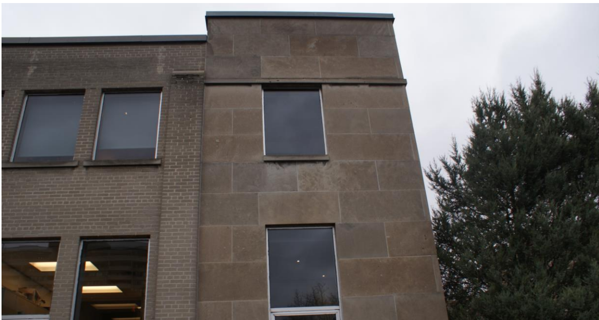
Figure 15: Detail view of the east-side elevation. The stone cladding returns on the side elevations and the rear portions of the building are clad in brick. The building is a composite construction with steel columns embedded in the walls. Note the stone above the first-floor window extends beyond the window opening and is supported by the masonry below. This suggests a traditional load bearing cladding affixed to a concrete block backup wall. Steel shelf angles are located above the second-floor windows supporting the parapet belt course. Source: CHRML
