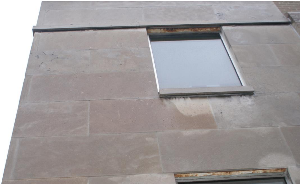
Figure 10: Note the rusting steel angle below the parapet belt course and the first floor window. There are indications on the north façade that the shelf angle below the parapet belt course is continuous. If this is the case, there is a high probability that the steel angle is secured to steel buried behind the wall (See Figure 13). Note the delaminating stone to the left of the second floor window and the discoloured stone below the window sill, which is an indication that the stone is being saturated by water from defective caulking. Source: CHRML.
