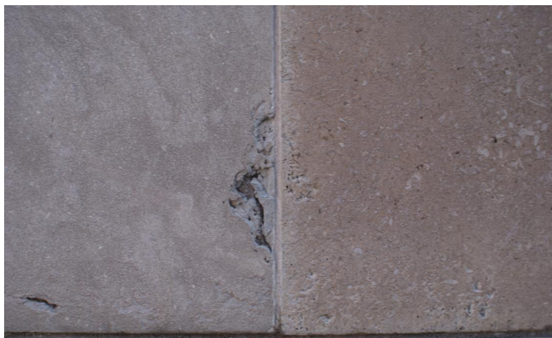
Figure 2: Detail view of ashlar limestone blocks. Note the voids or vugs in the unit to the left. Note the shell fragments in the block to the left. Source: CHRML.
