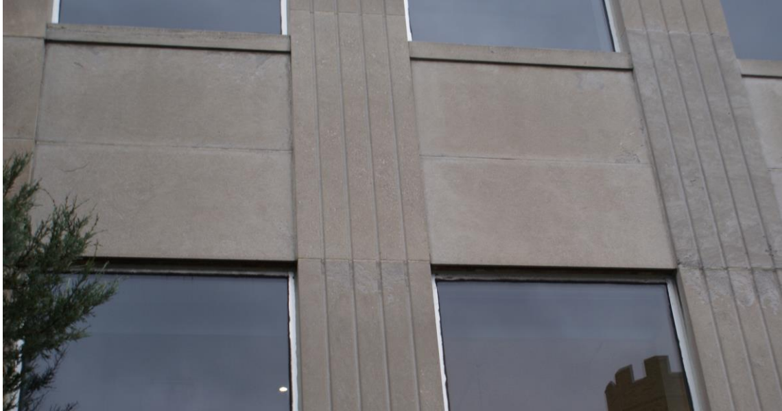
Figure 9: View of reeded stones where they meet at the top of the first floor windows. Note the chipping and scaling of the stones where they meet which may be due to compression failure. Source: CHRML.
