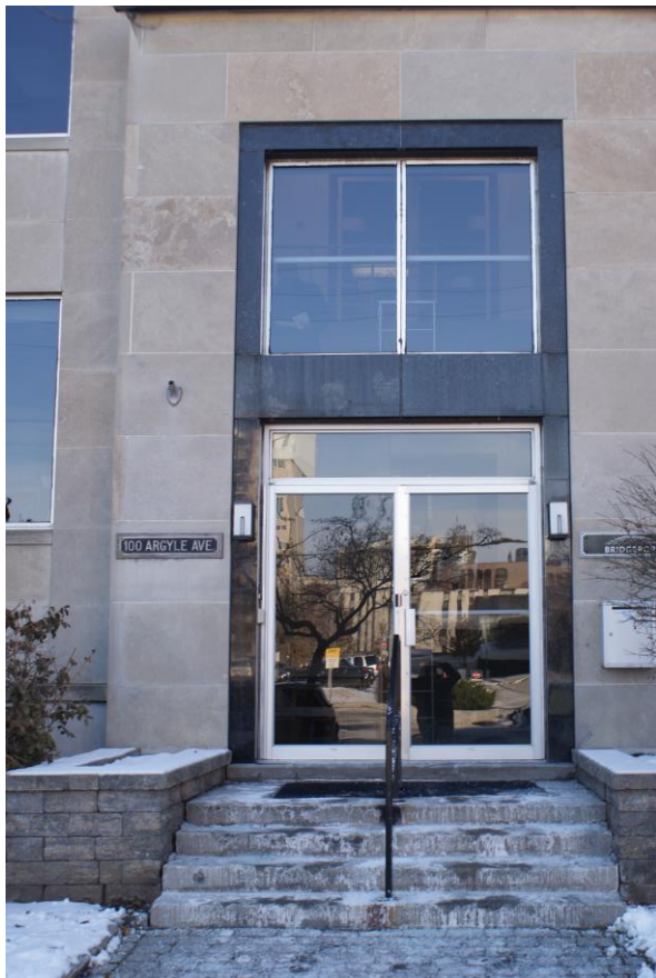
Figure 12: View of the main entrance to 100 Argyle. The entrance steps, doors, and upper transom are modern replacement units. The original entrance design is evident in the 1959 elevation drawings for the addition. Note the polished black granite entrance surround, street address plate and two sidelights all of which are original architectural features. The plan is to remove the stairs and drop the floor level to the same grade as the sidewalk to provide accessible access. Source: CHRML
