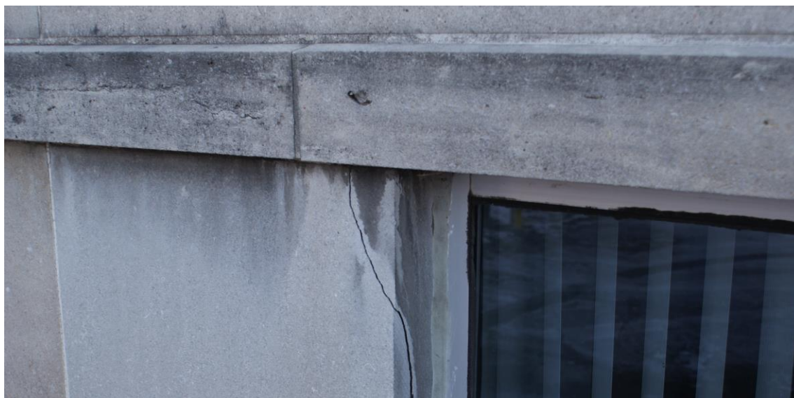
Figure 4: View of a stone in the belt course (left) that is in the process of fracturing at a bedding plane that has different material characteristics. Source: CHRML.
