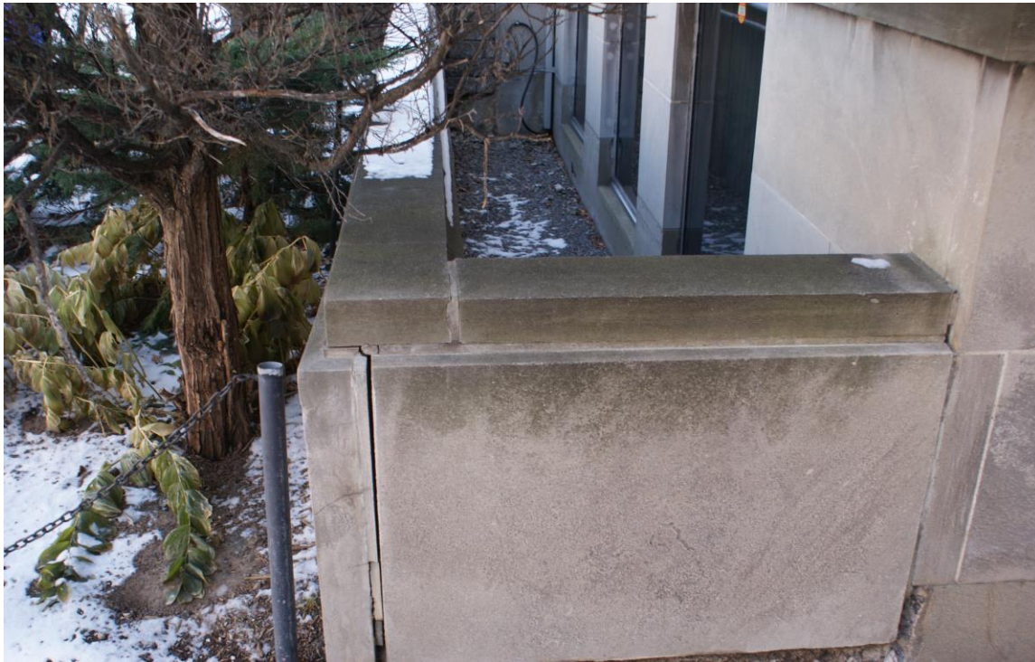
Figure 7: View of limestone clad area wall and coping. Note that the basement windows are set into the foundation wall. Source: CHRML.
