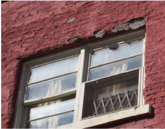
Photo 4 - Brick Spalling Above Window
