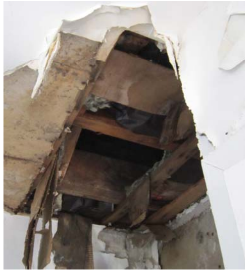
Photo 6 - Collapsed Ceiling and Water Damage
