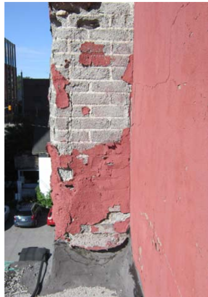
Photo 5 - Brick Spalling Above Roof
