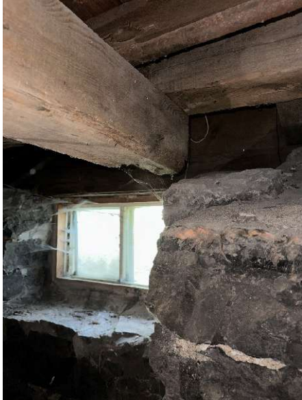
Photo 9: 281 Bell St - Primary ground floor beam shifted and unsupported
