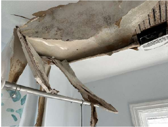
Phot 5: 281 Bell St - Interior Failed Ceiling
