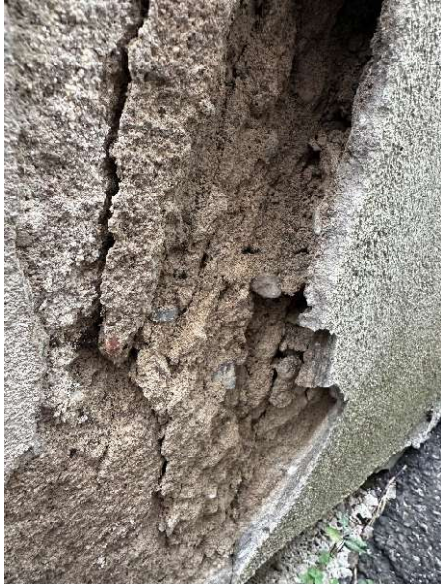
Photo 13: 275 Bell St - Concrete foundation deterioration (exterior)
