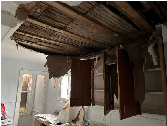
Photo 3: 281 Bell St - Failed Interior Ceiling
