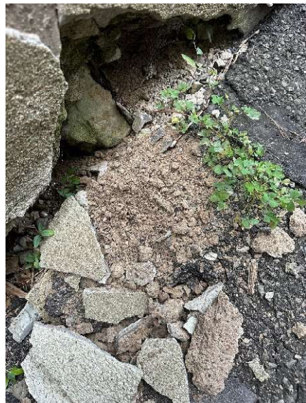
Photo 12: 273 Bell St - Concrete foundation deterioration at grade (exterior)
