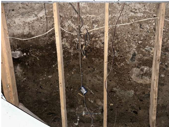
Photo 19: 275 Bell St - Foundation wall Water ingress and deterioration (interior)
