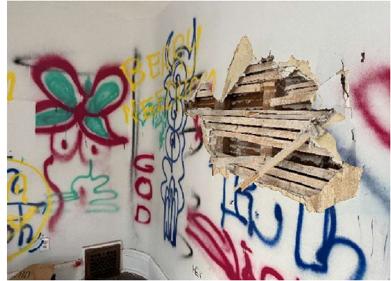
Photo 6: 281 Bell St - Interior wall damage
