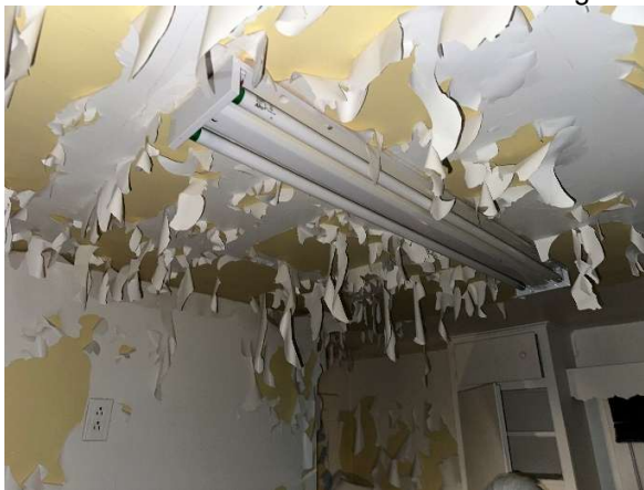
Photo 7: 277 Bell St - Interior finishes deterioration
