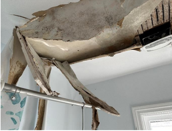
Phot 5: Interior Failed Ceiling
