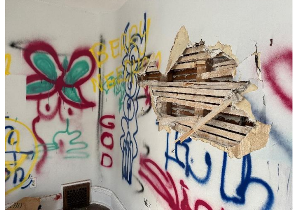
Photo 6: Interior wall damage
