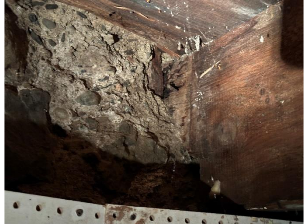
Photo 18: Wood beam Dry rot
