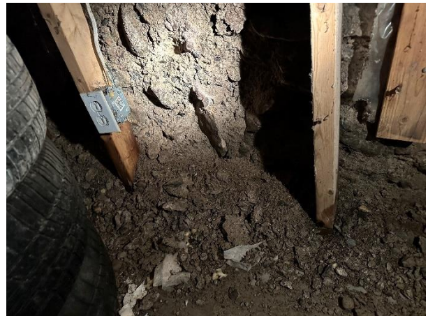
Photo 16: Concrete foundation deterioration (interior)
