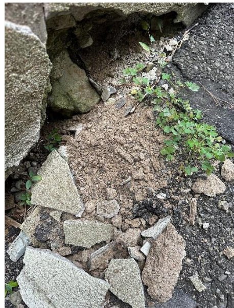
Photo 12: Concrete foundation deterioration at grade (exterior)
