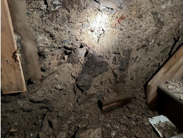
Photo 17: Concrete foundation deterioration (interior)
