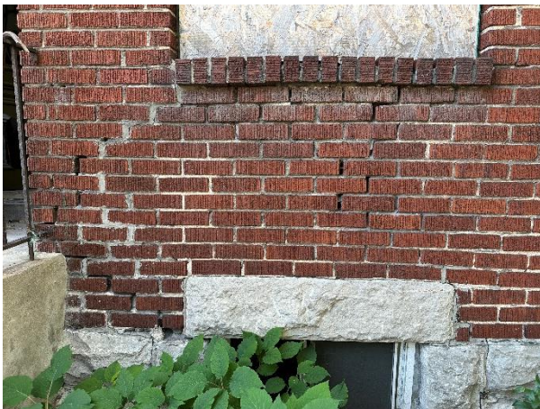
Photo 11: Exterior Brick damage – Step cracking
