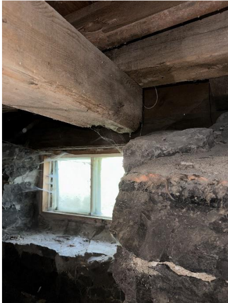
Photo 9: Primary ground floor beam shifted and unsupported
