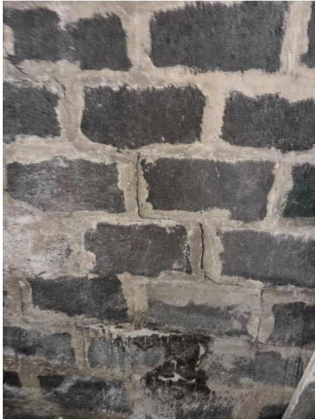
Photo 21: Step cracking in interior foundation wall
