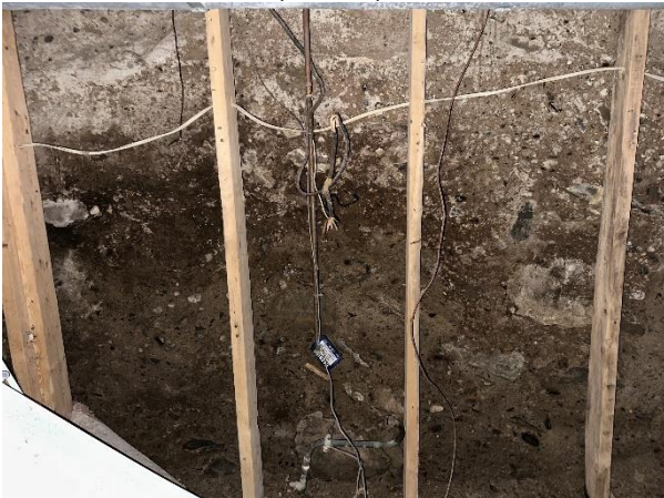
Photo 19: Foundation wall Water ingress and deterioration (interior)
