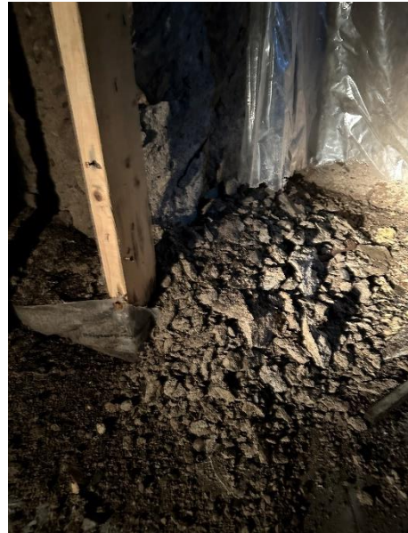
Photo 20: Foundation wall debris at base of wall (interior)
