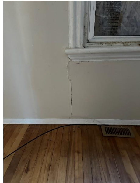
Photo 8: Interior cracking in finishes at window
