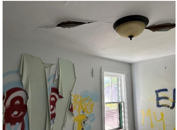
Photo 4: Interior paint peeling and ceiling damage
