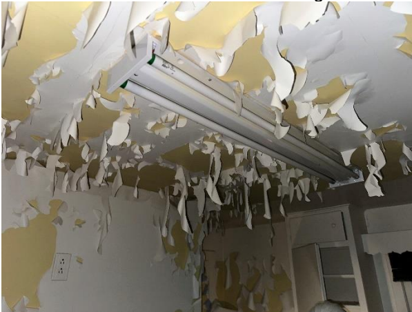
Photo 7: Interior finishes deterioration
