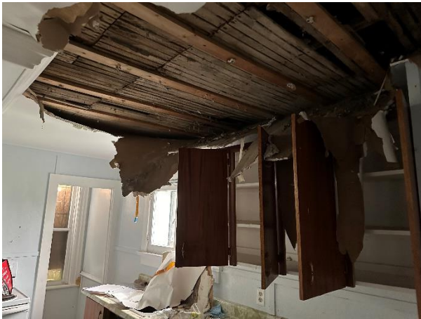
Photo 3: Failed Interior Ceiling
