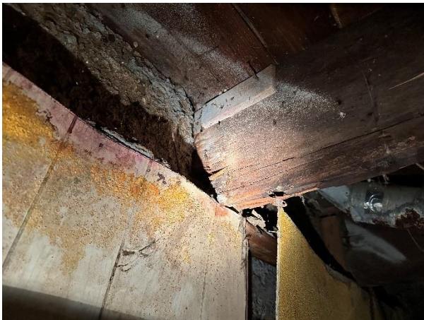
Photo 15: Unsupported wood floor beam
