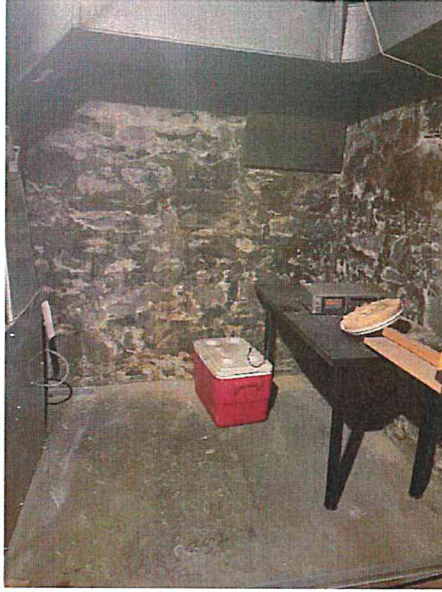
Typical Foundation Deterioration
