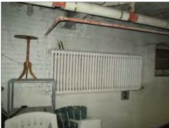
View of a typical hydronic, wall mounted radiator serving the UPG.
