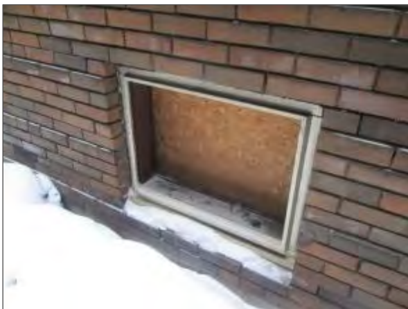
View of a missing window unit which has been covered with plywood on the north elevation of the building.
