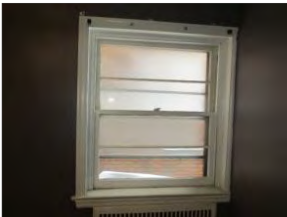
View of a typical older wood framed window serving the majority of the building.
