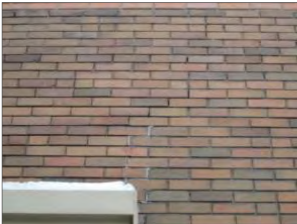
View of cracked masonry units and deteriorated mortar joints noted in the brick masonry on the west elevation of the building.
