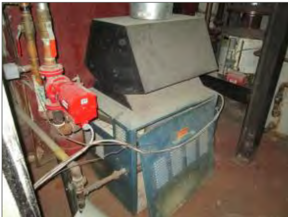
View of the second heating boiler serving the Site Building.
