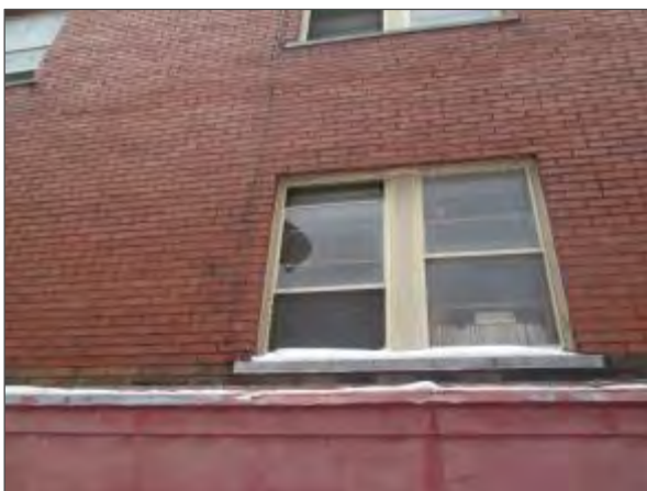
View of a cracked glazing unit noted on a storm window on the east elevation of the building.
