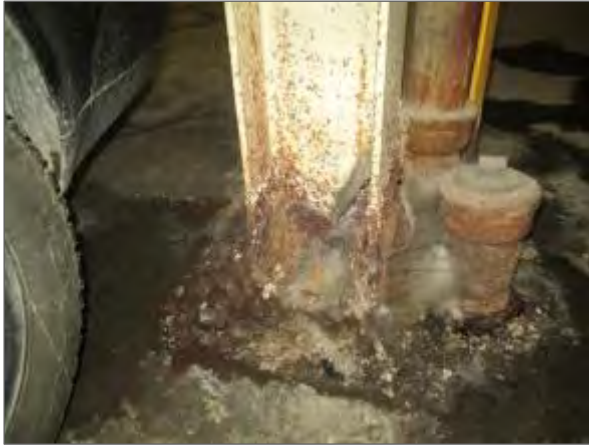
View of severe corrosion noted at the base of a column within the UPG.
