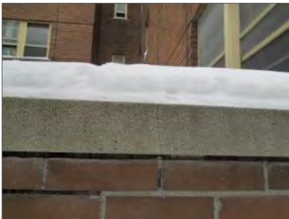
View of a small crack noted in a concrete coping stone on the south elevation of the building.
