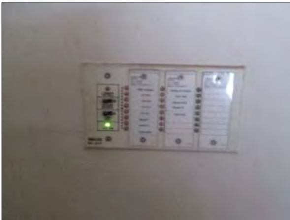
View of the annunciator panel which is located in the main entrance lobby area.
