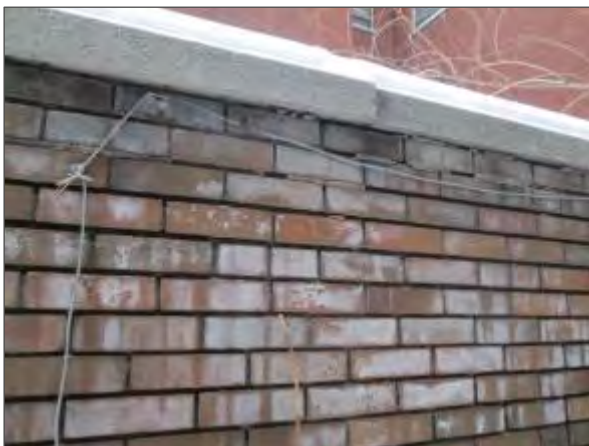
View of deteriorated mortar joints, efflorescence and a displaced concrete coping stone noted on the portion of the exterior wall which is slightly bulged.
