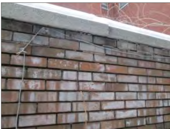
View of deteriorated mortar joints, efflorescence and a displaced concrete coping stone noted on the portion of the exterior wall which is slightly bulged.
