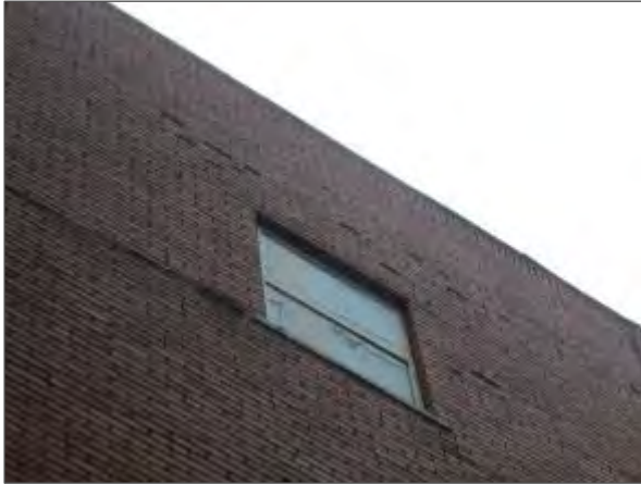
View of spalled brick masonry units noted at the top of the east elevation of the building.
