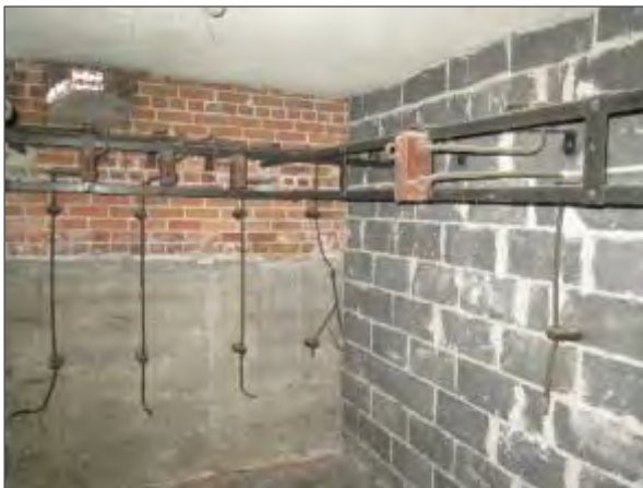
View of the abandoned knob and tube wiring system noted in the former main electrical room.
