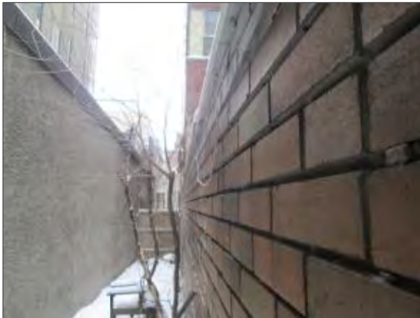
View of an area of brick masonry on the north elevation of the building (wall which flanks the UPG) which has a slight bulge.
