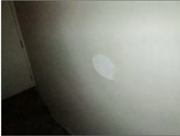
View of popping plaster finishes noted within a stairwell.
