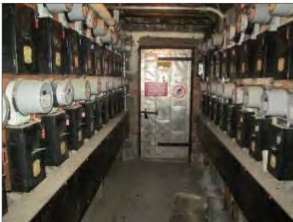
General view of the main electrical room in the basement of the building.
