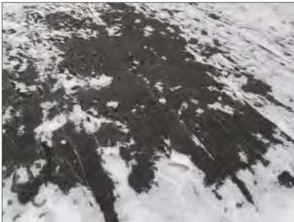
View of cracking and deterioration noted in the mop-on membrane on the north UPG roof.
