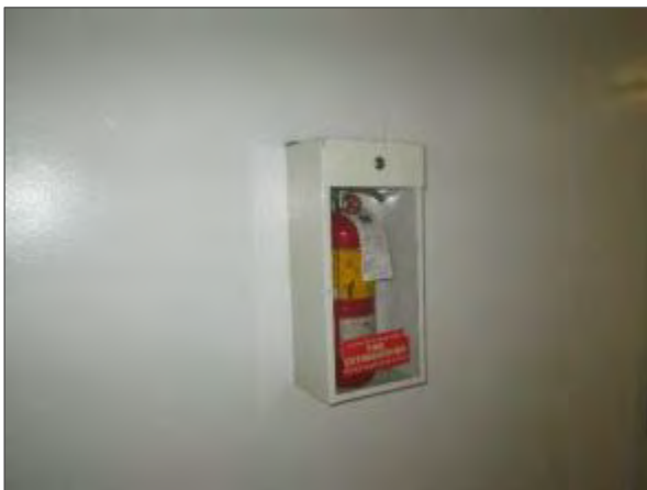
View of the typical cabinet mounted chemical fire extinguishers serving the Site Building.
