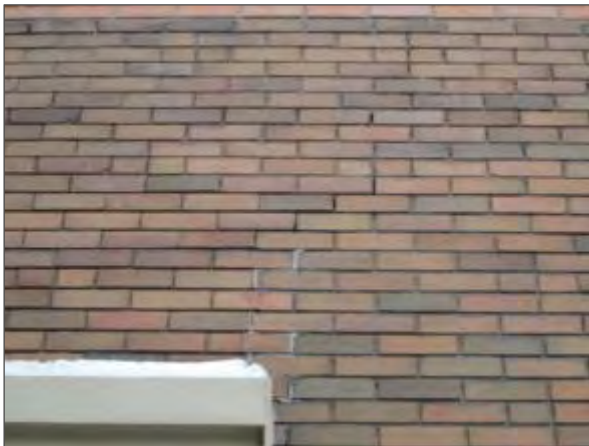
View of cracked masonry units and deteriorated mortar joints noted in the brick masonry on the west elevation of the building.
