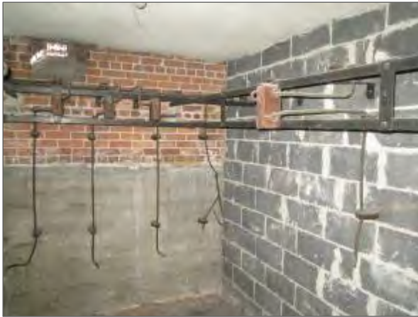
View of a combination cast-in-place concrete and solid brick masonry foundation wall as well as a typical cinder block masonry demising wall.
