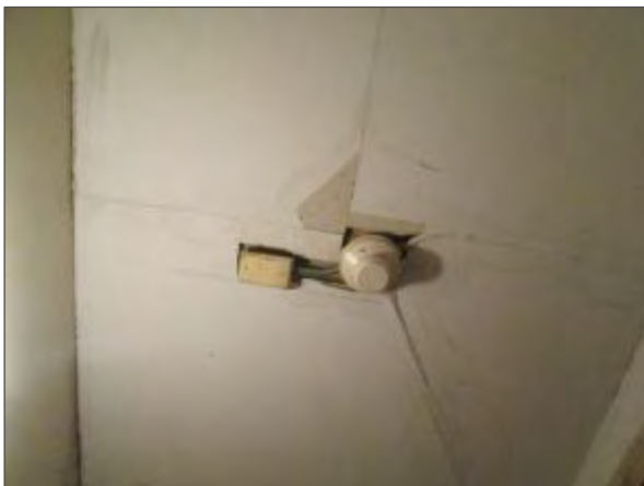
View of damaged gypsum ceiling finishes noted near the roof access door.
