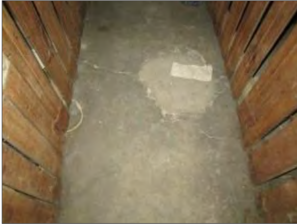
View of cracking noted in the concrete floor slab in a basement locker room.
