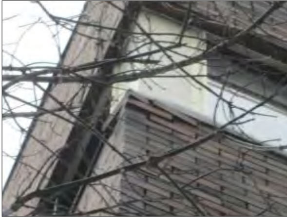
View of loose brick masonry units noted on the south elevation of the building.
