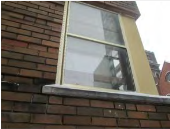
View of a cracked glazing unit noted on a storm window on the north elevation.
