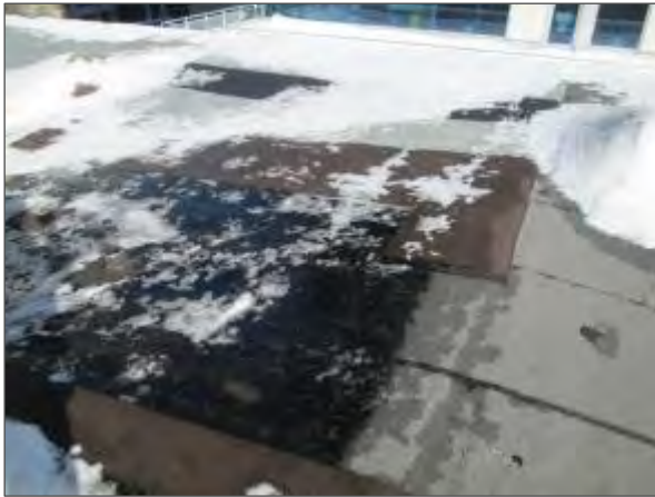
View of several patch repairs noted on the main roof of the building atop the fourth floor.
