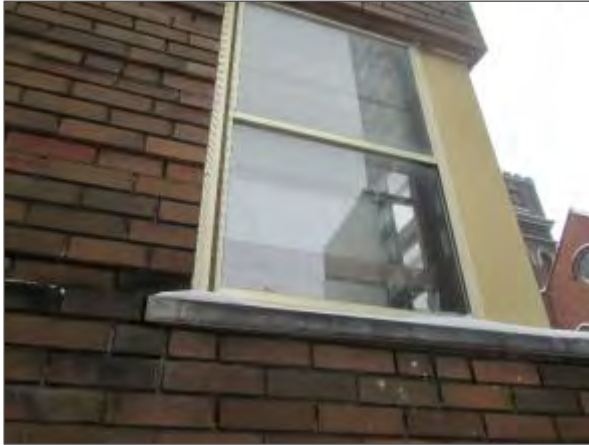
View of a cracked glazing unit noted on a storm window on the north elevation.
