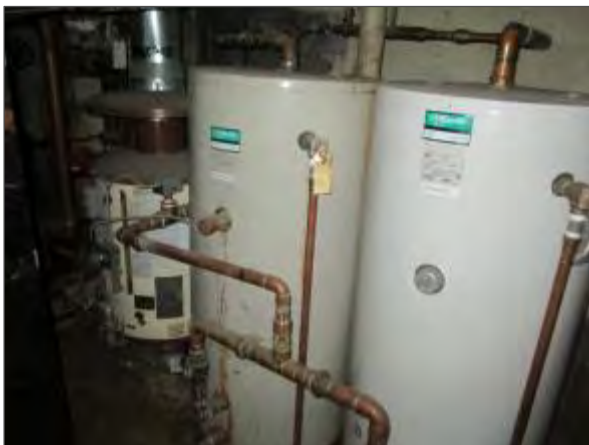
View of the DHW boiler and the two associated storage tanks.
