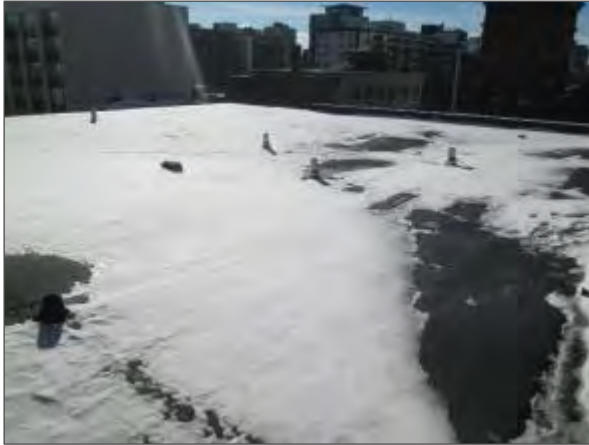
View of a portion of the main roof system atop the fourth floor of the building.
