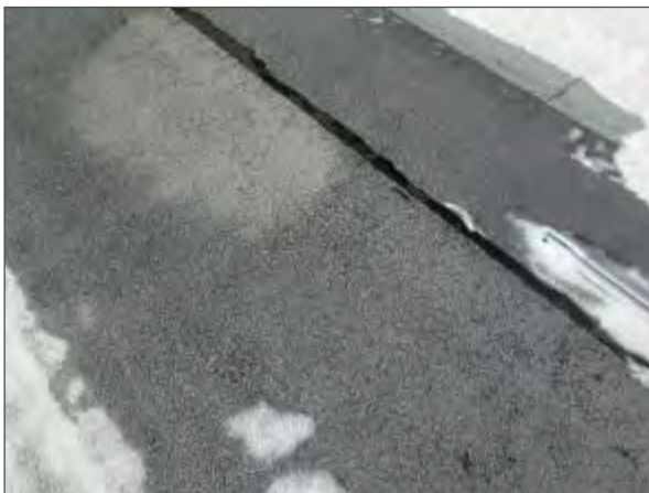
View of crazing and deterioration noted in a section of modified bitumen membrane atop the fourth floor roof.
