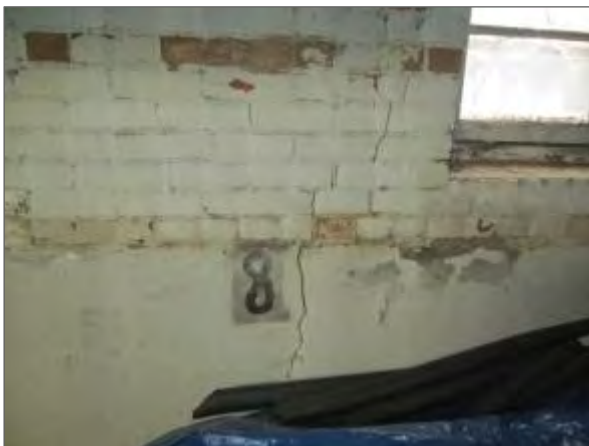
View of cracking noted in the cast-in-place concrete and brick masonry foundation walls on the south portion of the UPG.
