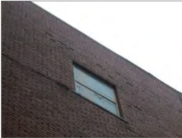
View of spalled brick masonry units noted at the top of the east elevation of the building.
