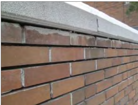
View of deteriorated mortar joints noted within the brick masonry on the south elevation of the building.
