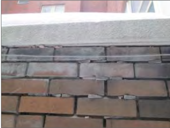
View of deteriorated mortar joints noted in the brick masonry on the south elevation and a crack in the concrete coping stone.
