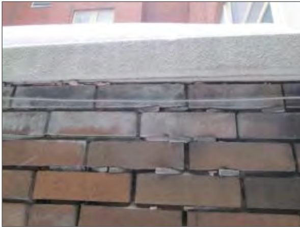
View of deteriorated mortar joints noted in the brick masonry on the south elevation and a crack in the concrete coping stone.
