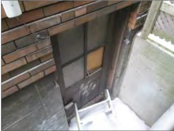
View of the old and damaged secondary access door to the boiler room which is reportedly no longer used.
