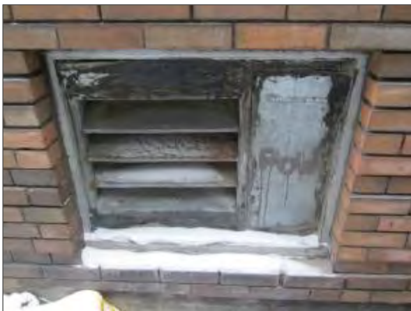
View of faded paint finishes and deteriorated sealants on the boiler room ventilation louver.
