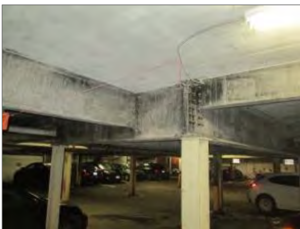
View of the steel beams and columns located in the UPG of the building which support the central portion of the building.
