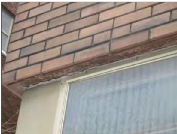
View of corrosion on a window lintel and a deteriorated perimeter window sealant observed on the south elevation of the building.
