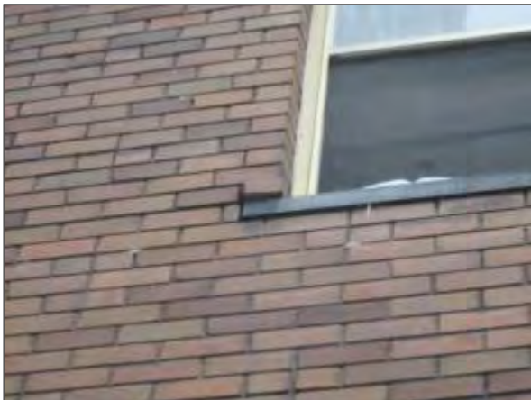
View of a loose brick masonry unit noted on the west elevation of the building.
