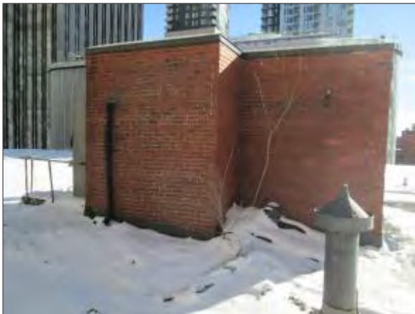
View of vegetative growth noted near the exterior wall of the stairwell penthouse on the main roof.
