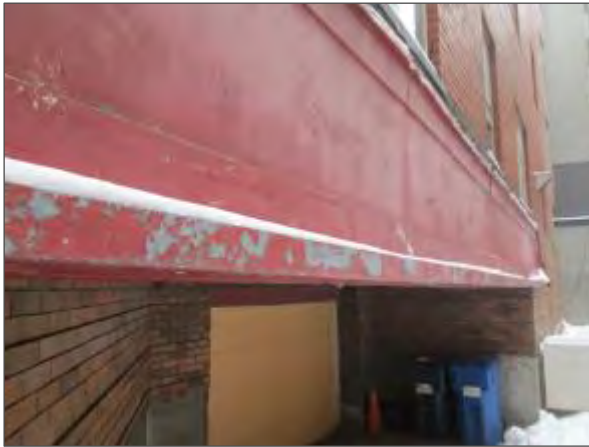
View of deteriorated paint finishes noted on the metal cladding above the overhead door serving the UPG on the east elevation of the building.
