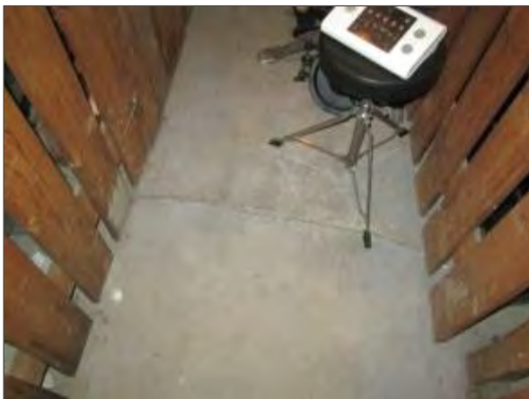
View of cracking noted in the concrete floor slab in a basement locker room.
