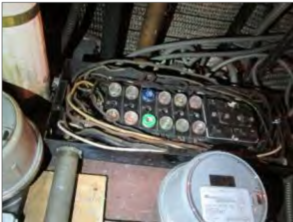
View of a glass plug fuse electrical panel noted in the main electrical room.
