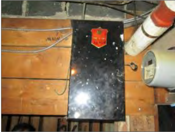
View of the original main disconnect switch serving the Site Building.
