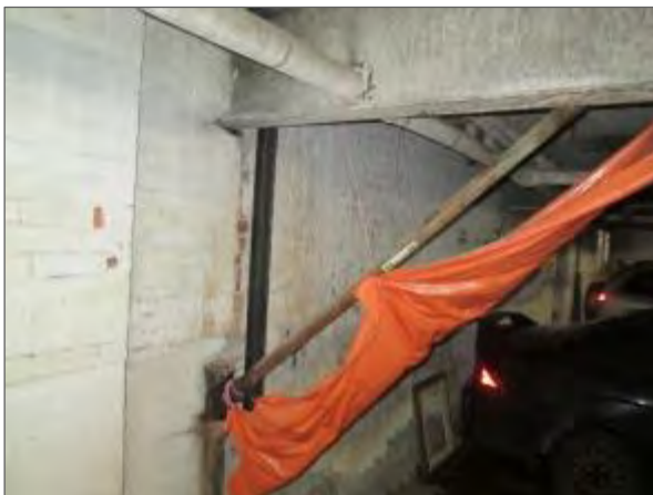
View of an orange tarp which is being used to divert leaking water from the UPG roof deck to the perimeter of the UPG.
