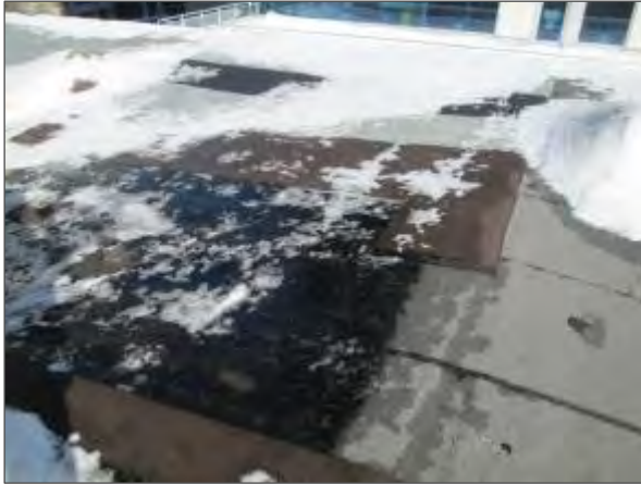
View of several patch repairs noted on the main roof of the building atop the fourth floor.
