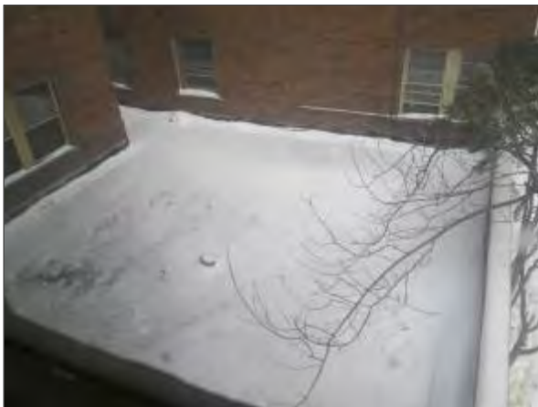
View of the snow covered roof system atop the UPG roof on the south portion of the building.
