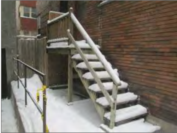
View of the wood framed staircase located on the north elevation of the building.
