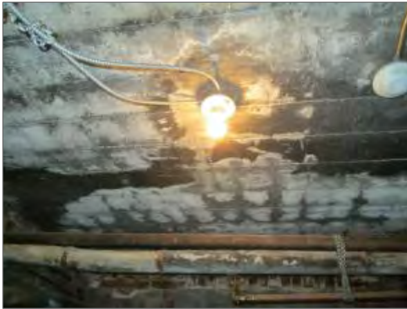
View of efflorescence noted on the soffit of the UPG roof deck within a service room in the northwest portion of the UPG.
