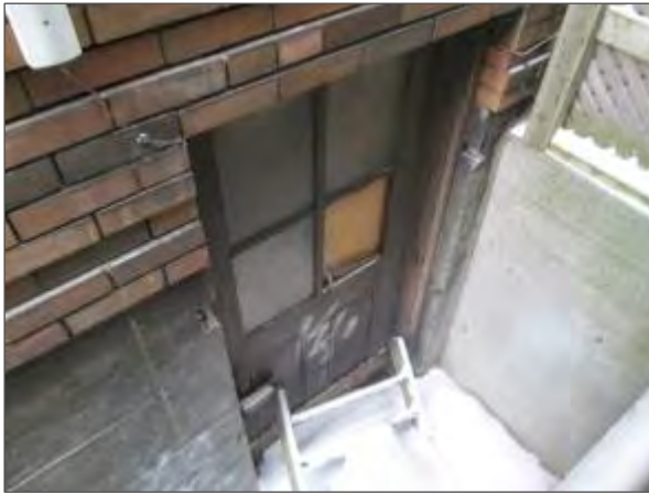
View of the old and damaged secondary access door to the boiler room which is reportedly no longer used.
