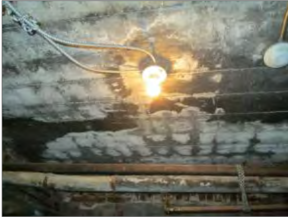
View of efflorescence noted on the soffit of the UPG roof deck within a service room in the northwest portion of the UPG.
