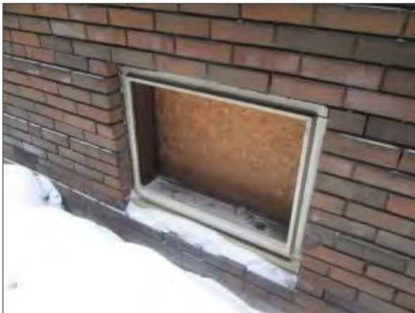
View of a missing window unit which has been covered with plywood on the north elevation of the building.
