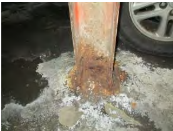
View of severe corrosion noted at the base of a column within the UPG.
