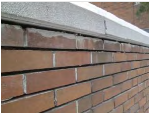
View of deteriorated mortar joints noted within the brick masonry on the south elevation of the building.
