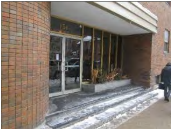
View of the terrazzo staircase serving the main entrance of the building on the west elevation.
