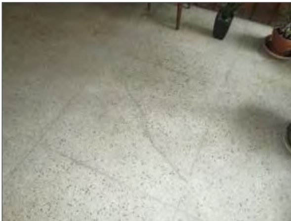
View of cracked terrazzo flooring noted in the main entrance lobby.
