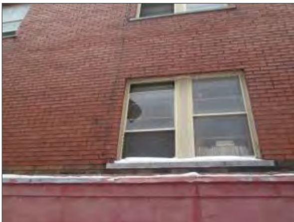
View of a cracked glazing unit noted on a storm window on the east elevation of the building.
