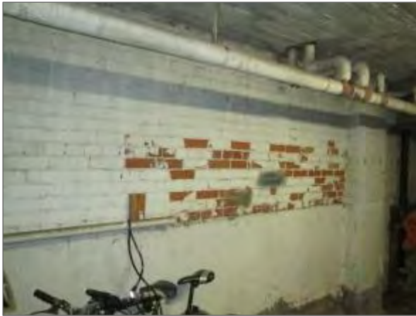
View of spalling brick masonry noted on the south foundation wall of the UPG.
