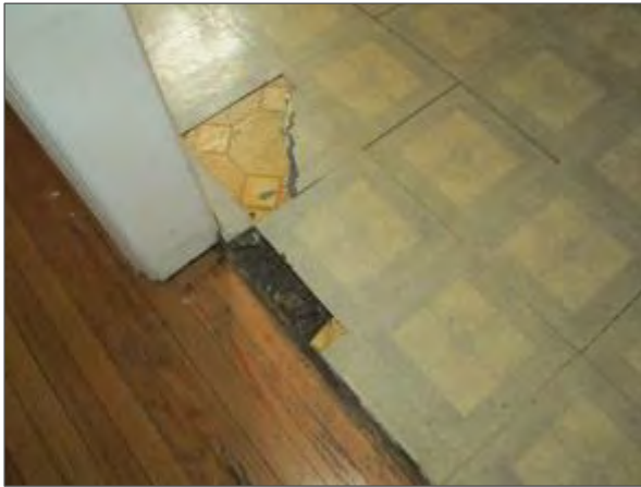
View of damaged vinyl floor tiles noted within the kitchen of suite 204.
