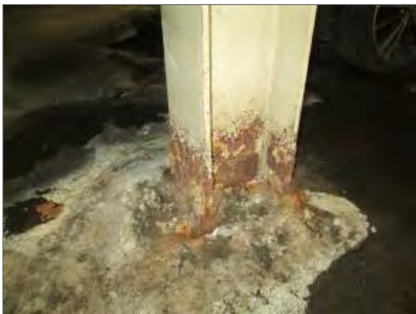
View of severe corrosion noted at the base of a column within the UPG.
