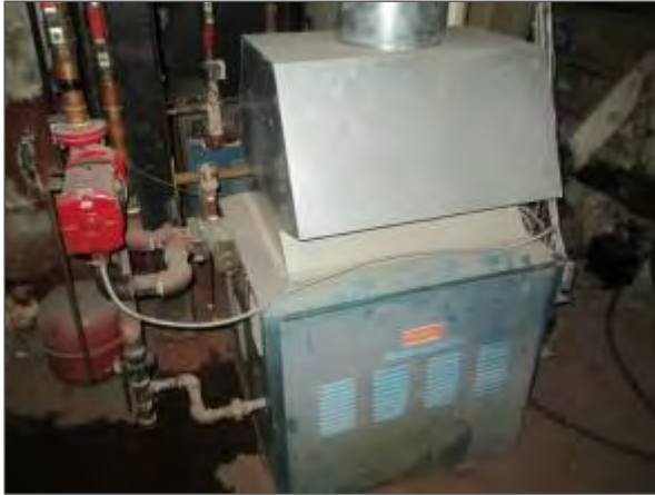
View of the first heating boiler serving the Site Building.
