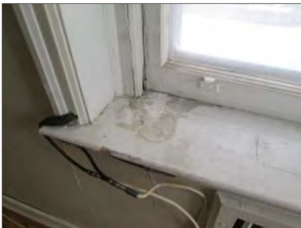
View of a damaged wood window sill noted in suite 204.
