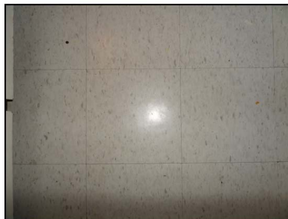
Photograph 2 - Flooring NON-DETECT for asbestos. TOP: 12”x12” vinyl floor tiles (light beige with blue streaks) from the Kitchen at 1-145 Arlington Avenue. BOTTOM: 12’x12” vinyl floor tiles (light beige with brown specks) from the Kitchen at 2-145 Arlington Avenue.
